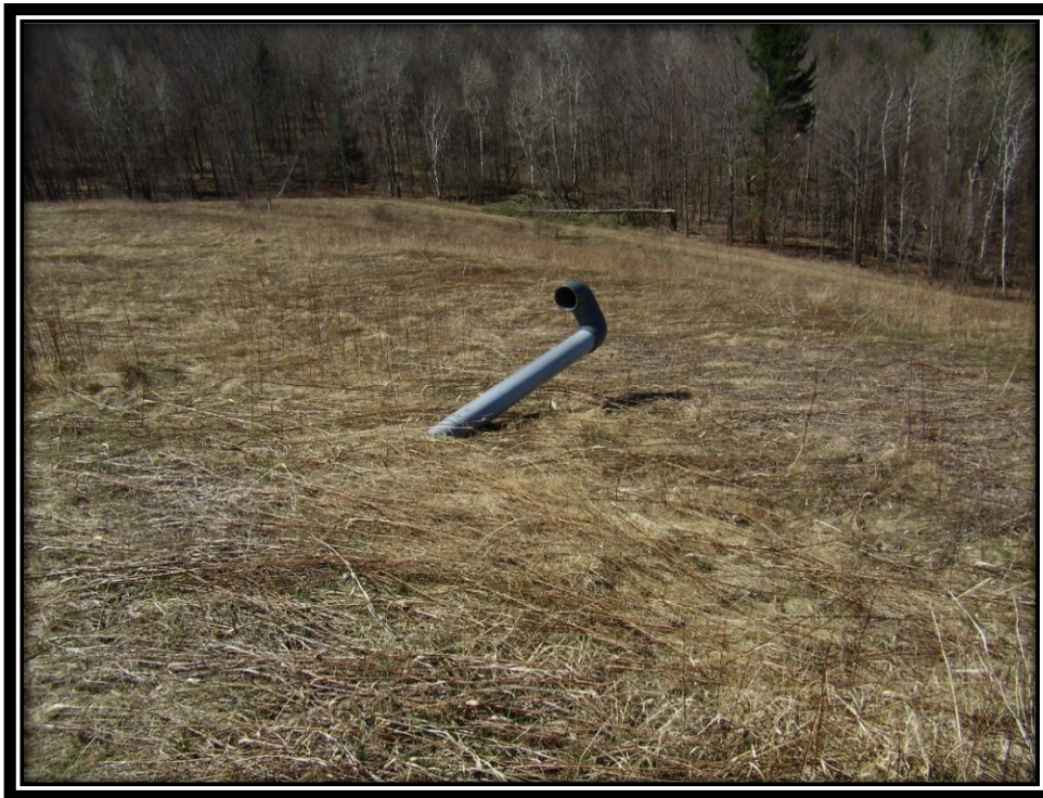
Photo 11: Broken gas well requiring repair. This is the only well, of approximately eight passive gas wells, that appeared to have any damage.
