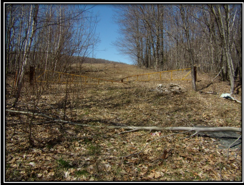
Photo 1: Entrance gate to the landfill. The gate is in poor condition but still effective in preventing vehicular access, however, the site is also accessible from at least one other location.
