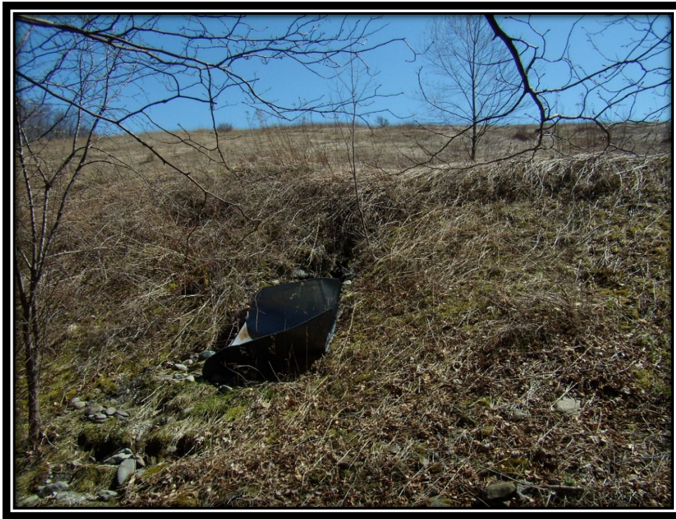
Photo 10: Several maintenance issues were identified at the site such as this culvert exit point that had a dislodged diffuser. Another culvert approximately 100 feet north of this location had the same condition.
