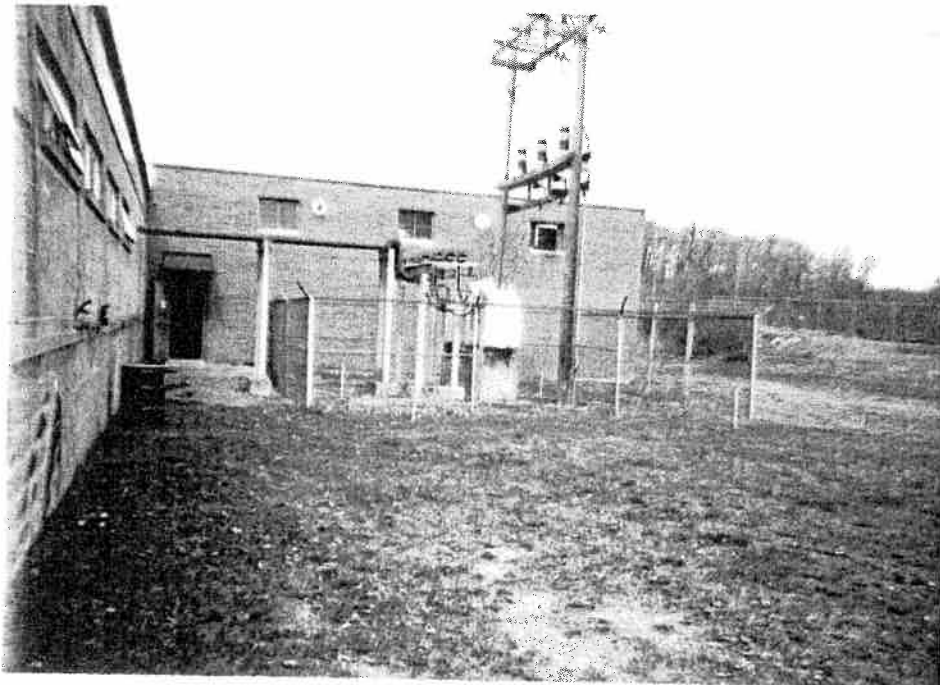
2. View northeast. NMPC transformer pad.
