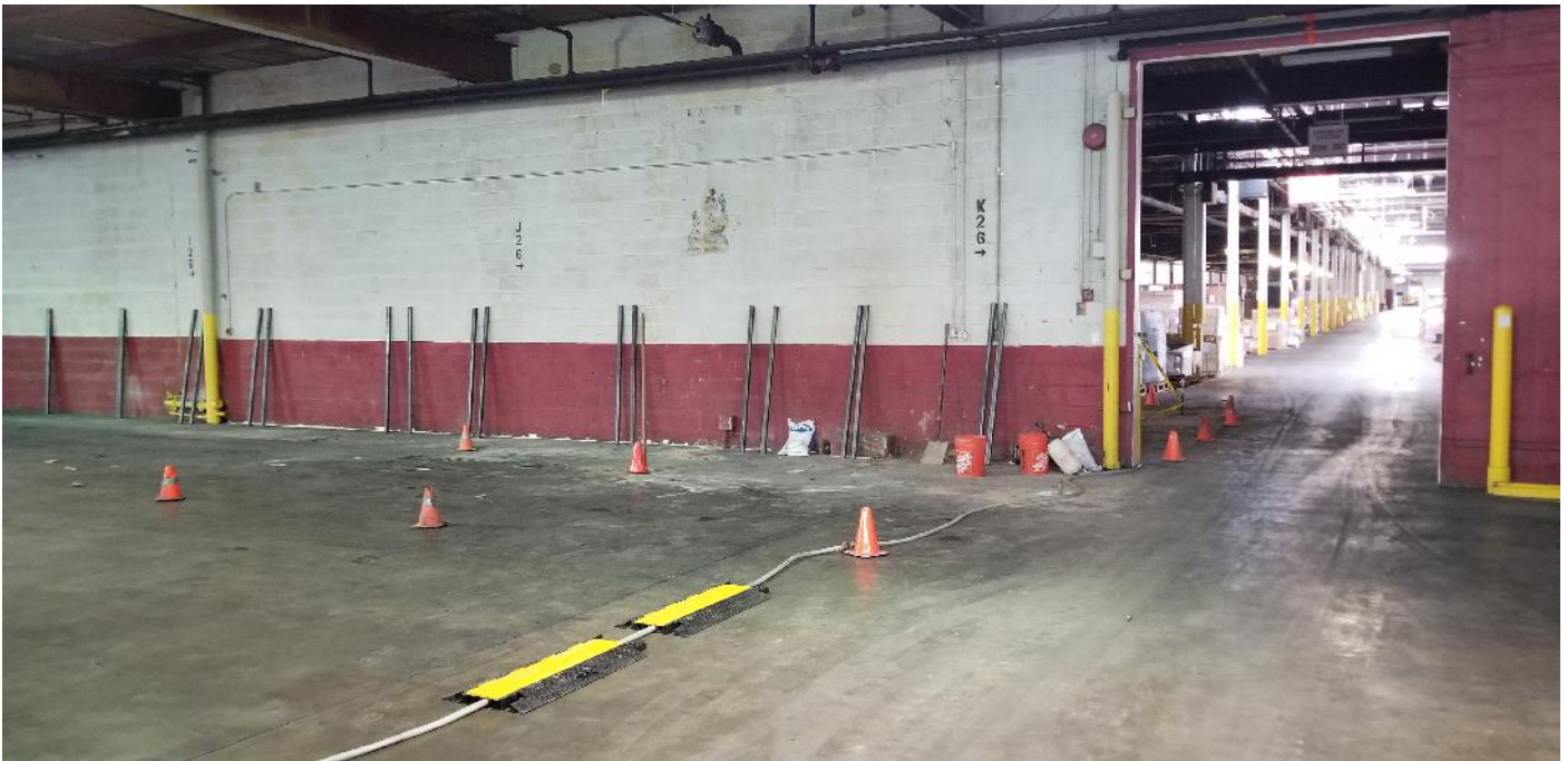
Picture 5: Building #61 ISCO injection area; north of well MP-37 (view looking south)
