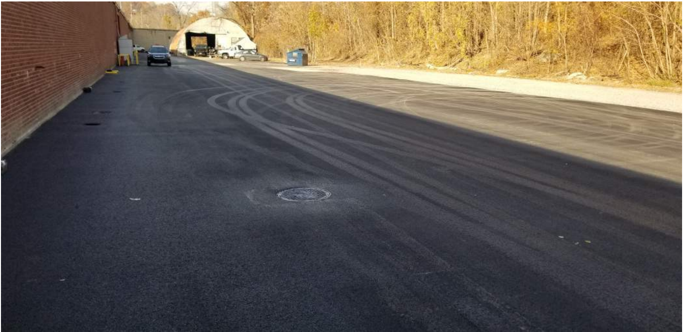
Figure 7. Paved parking area north of Building #61; sewer manhole MH-2 in foreground (view looking west).
