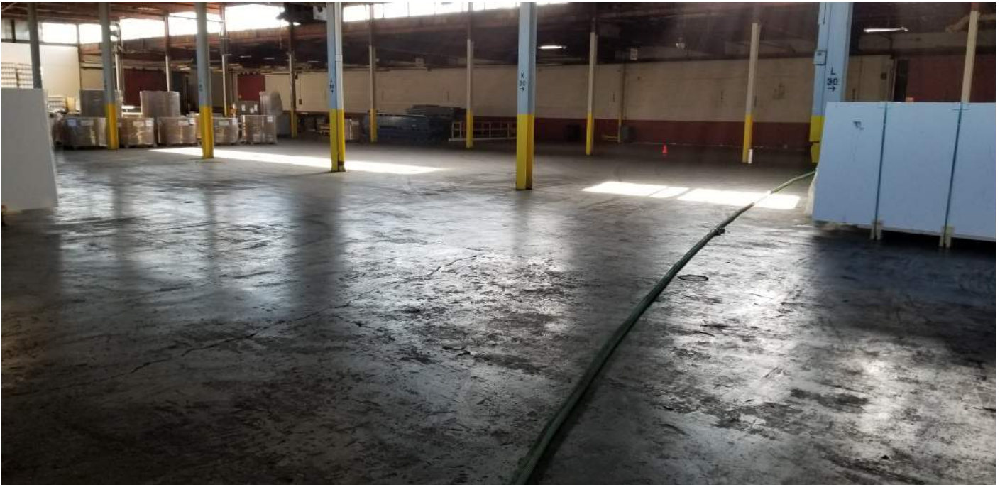
Figure 17. Concrete slab in Building #61; traffic cone at monitoring well MW-22 (view looking southeast)
