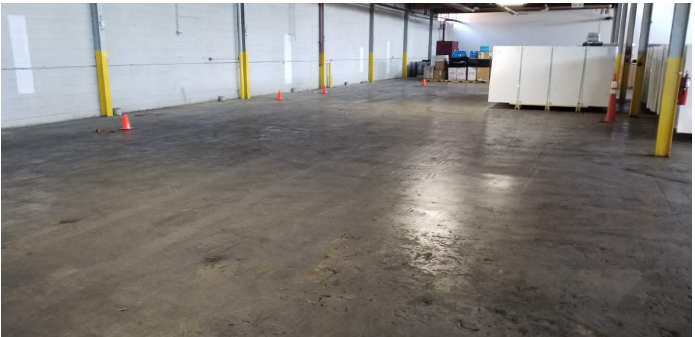
Figure 16. Concrete slab inside the northern portion of Building #61; traffic cones at monitoring wells MW-20, MP-26, MP-27, and MP-28 (left to right) (view looking northeast)
