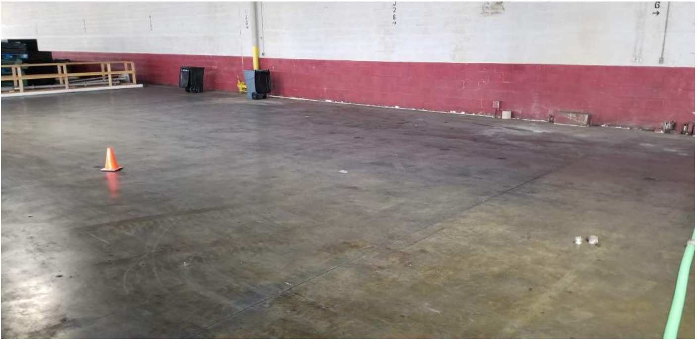
Figure 19. Concrete slab in Building #61; traffic cone at monitoring well MW-22 (view looking southeast)
