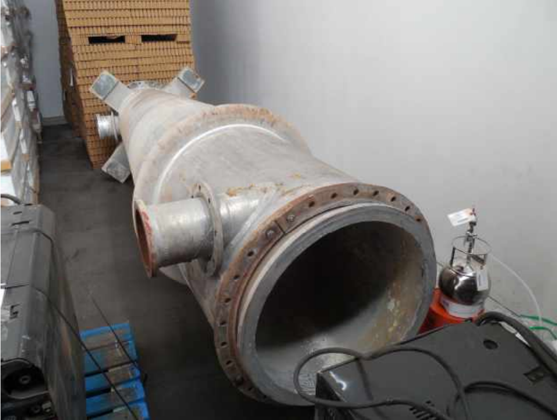
Picture 1: Steel stack/vent (Photoionization Detector [PID]: 1,275 – 1,252 parts per billion by volume [ppbv]) DB-VMP-2 in foreground.
