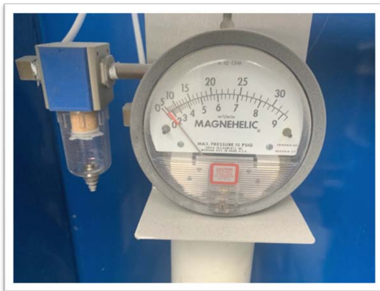
4. CFM Reading at the SVE System Unit
