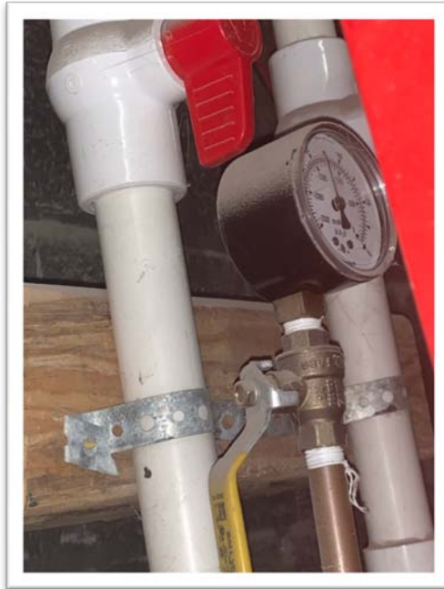
5. Vacuum Gauge of the SVE System in the Repair Shop Area
