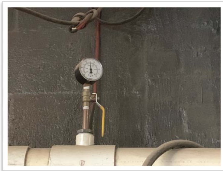
6. Vacuum Gauge of the SVE System in the Repair Shop Area
