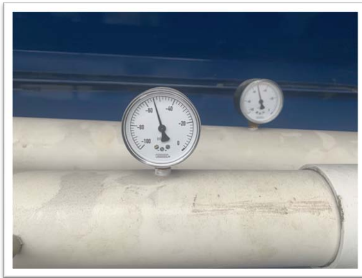
7. Vacuum Gauges of the SVE System Unit
