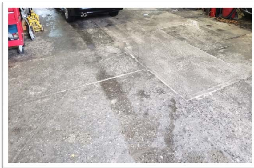
12. A View from the Interior Portion of the Site (SVE Wells Location - Sub-Slab)
