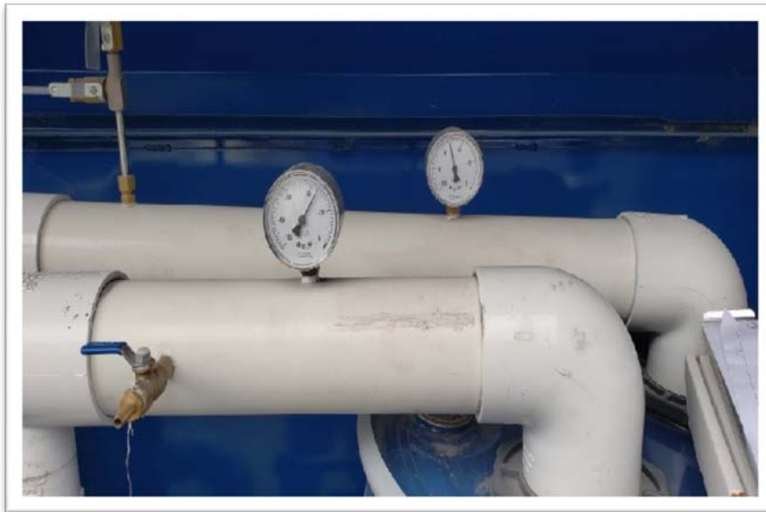
8. Vacuum Gauges of the SVE System Unit
