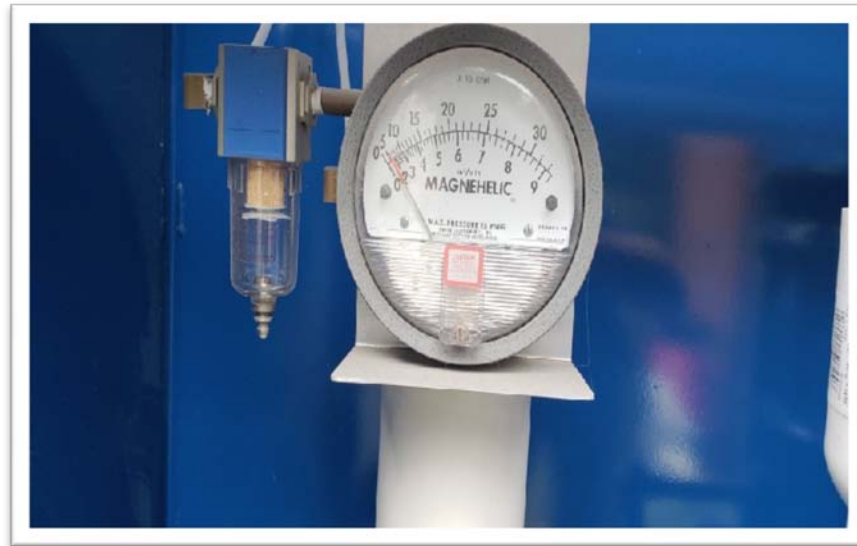
5. CFM Reading at the SVE System Unit
