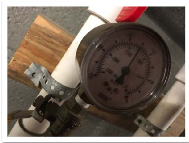
7. Vacuum Gauge of the SVE System in the Repair Shop Area
