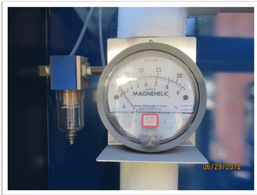
5. CFM Reading at the SVE System Unit
