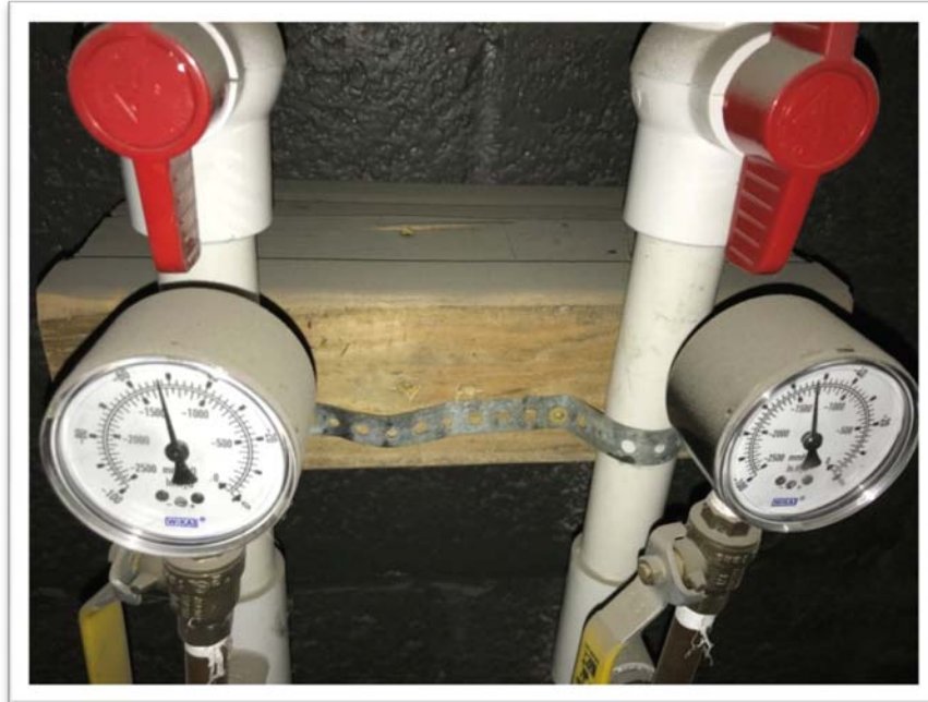
6. Vacuum Gauges of the SVE System in the Repair Shop Area
