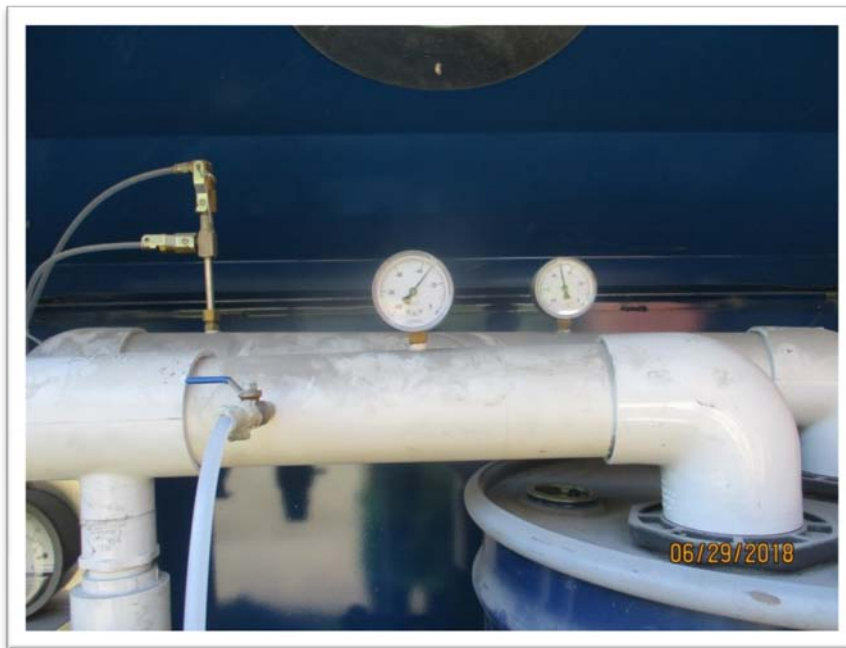
8. Vacuum Gauges of the SVE System Unit
