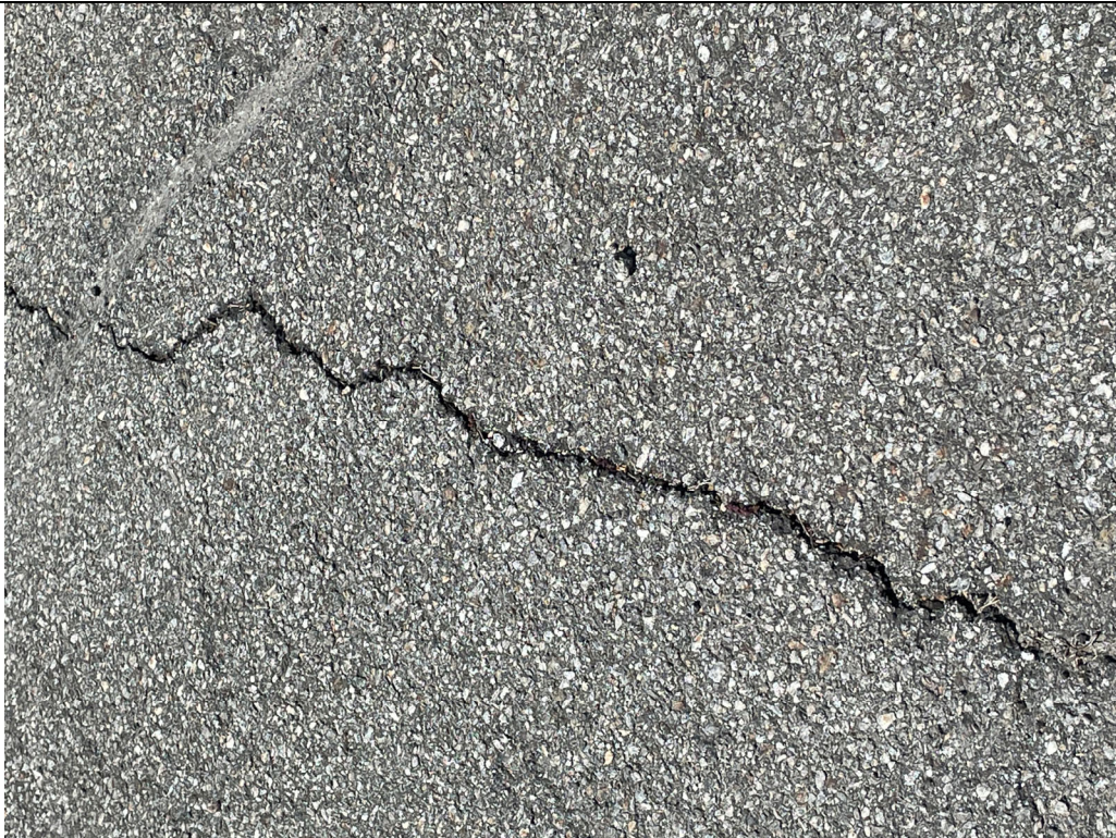
Crack in asphalt cover of OU-1
