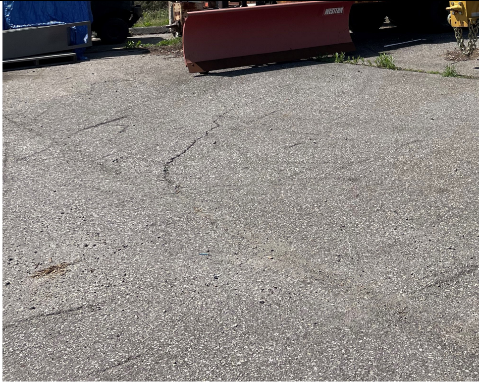
Cracks in asphalt cover of OU-1
