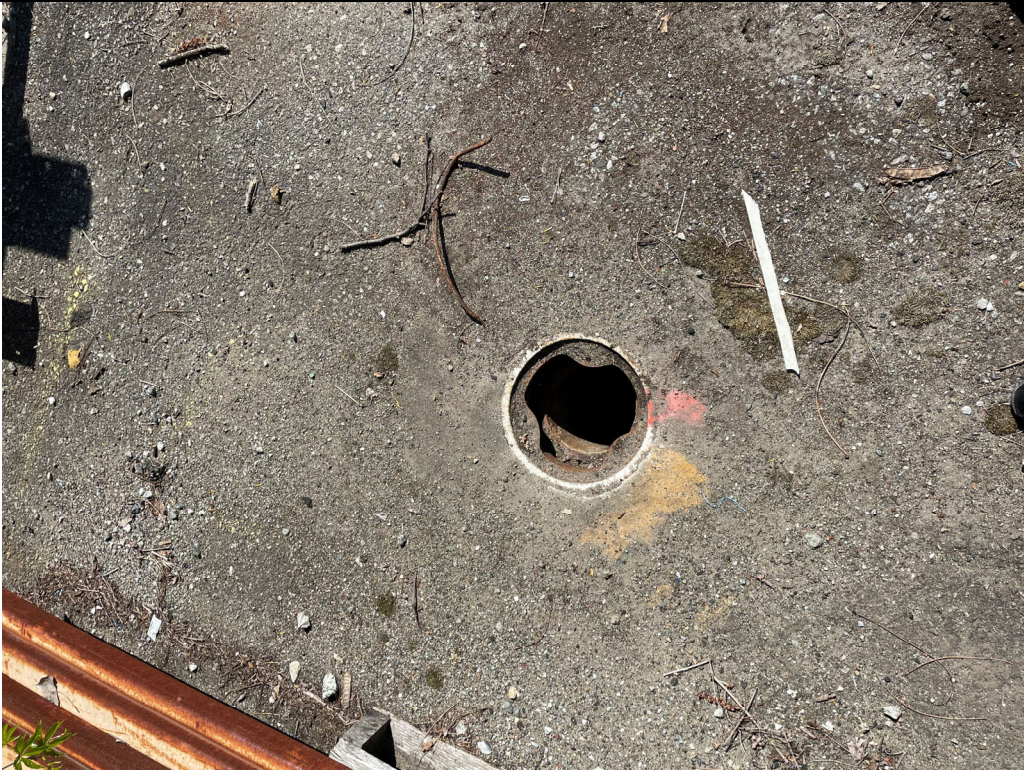
Missing cap of well P-7
