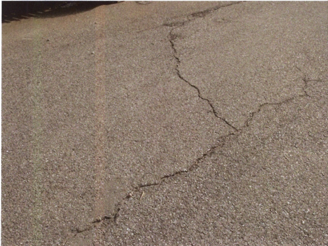
Picture #3 (12/17/08) Minor cracks that appear stabilized on asphalt cover.
