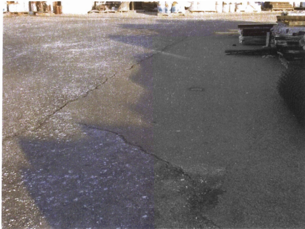
Surficial cracking observed throughout asphalt cover.
