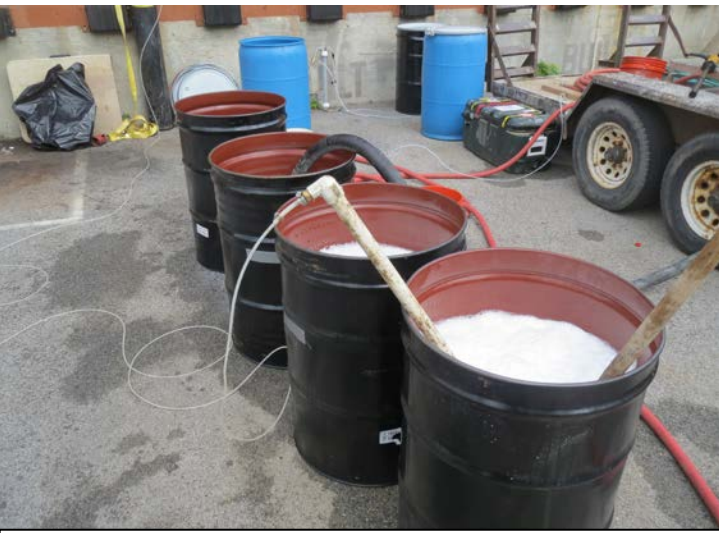
Photograph No. 5: Mixing 3D ME and HRC Regeneration solutions prior to injection.
