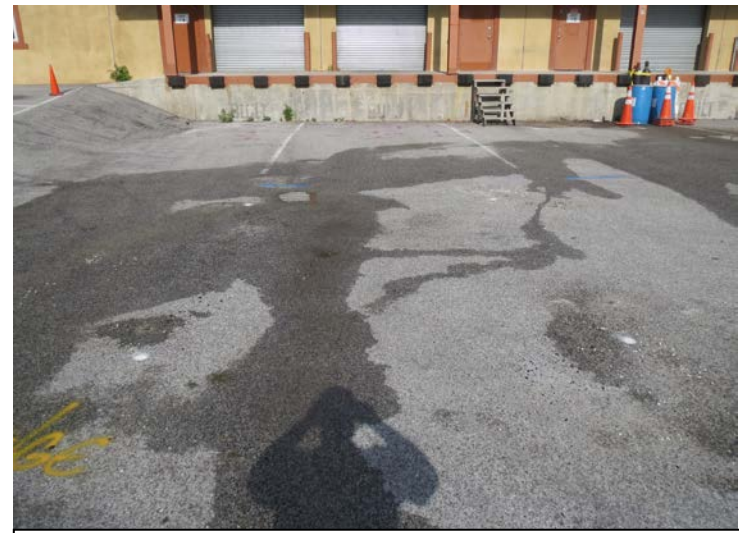
Photograph No. 6: Loading area after completion of bioremediation injection activities. White points indicate injection locations.
