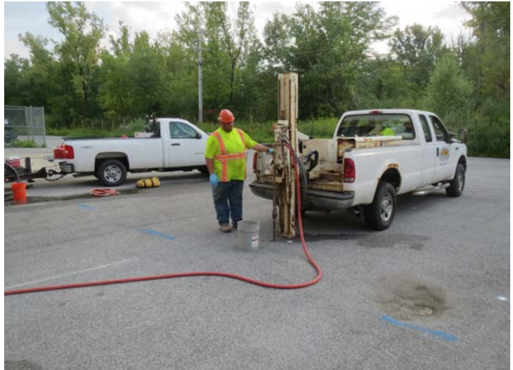
Photograph No. 4: Injecting bioremediation solution at IP4. Monitoring well MW-5A/AR north of IP 4 in photo.
