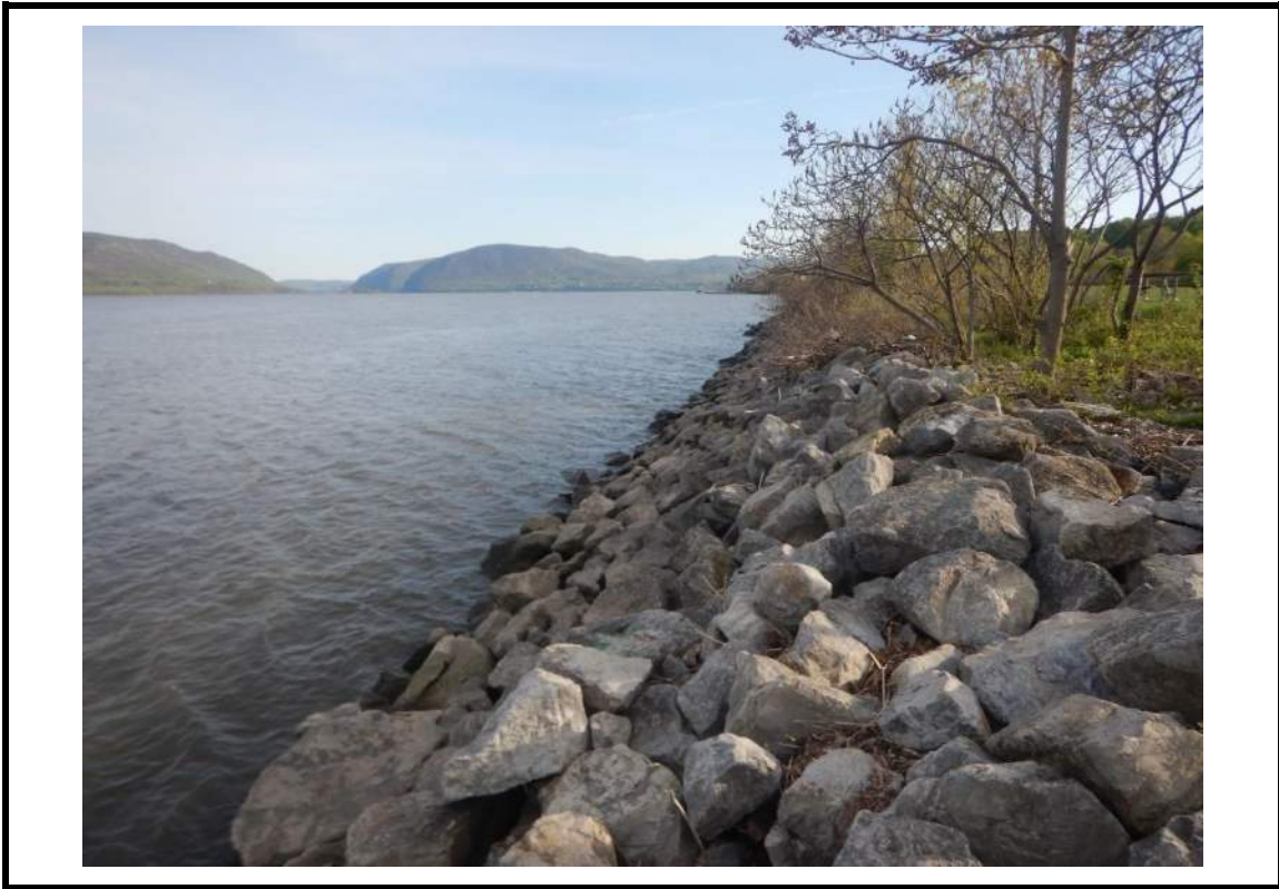
Photo #7 Description: View of eastern Site area, facing southeast, and rip-rap erosion blanket installed along Hudson River frontage.
