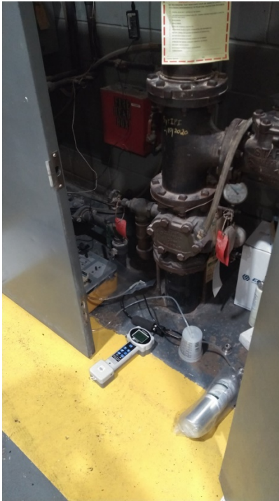
Photograph 5: Helium test pre sample collection fire closet
