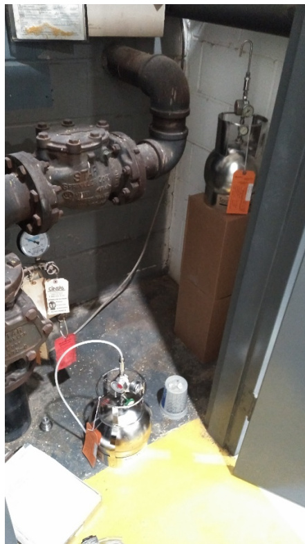
Photograph 4: Sprinkler room, SS-SV-06/IA-06
