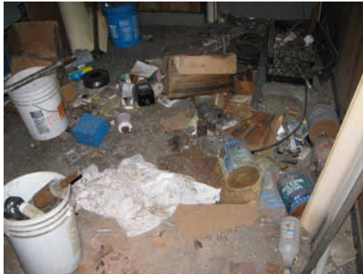
Typical building interior with containers of paints and other materials scattered with general garbage.
