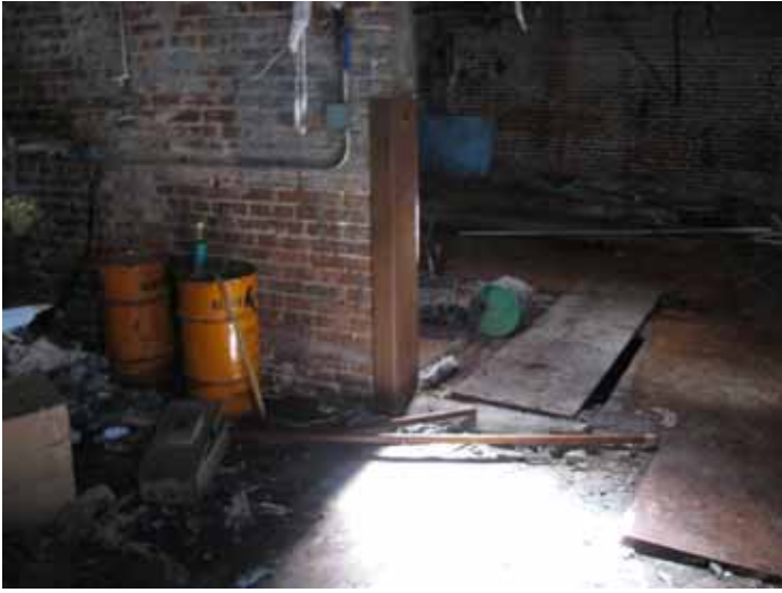
View of grease drums (left) and road plates at the entrance to the southern portion. The gap in the road plates is the location of a sump pit which is full of water.
