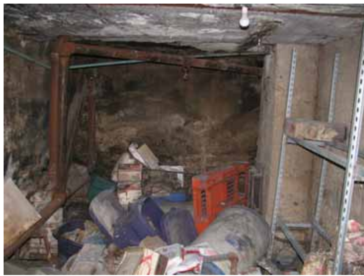
Interior of northern basement with drum and garbage on floor.
