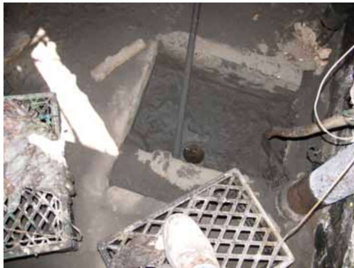
Sump in central basement with various pipes discharging to it and no known discharge point.
