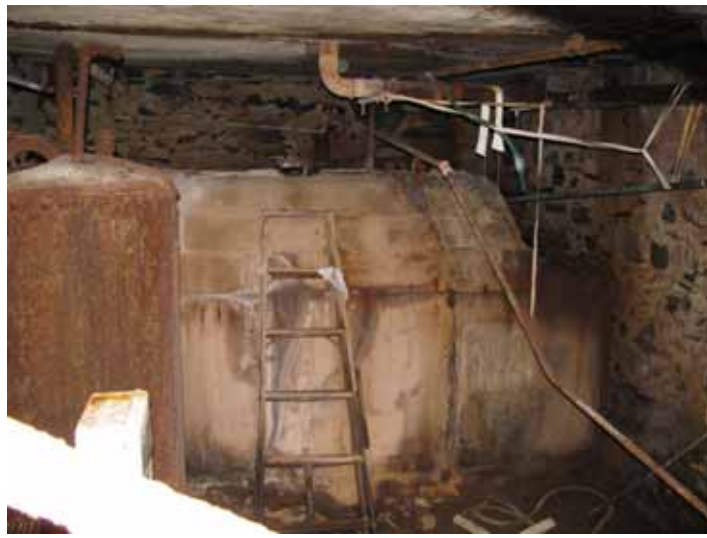
Vaulted AST in central basement. Note deaeration tank in foreground on left side and piping leading to the sump just off camera on the bottom right corner.
