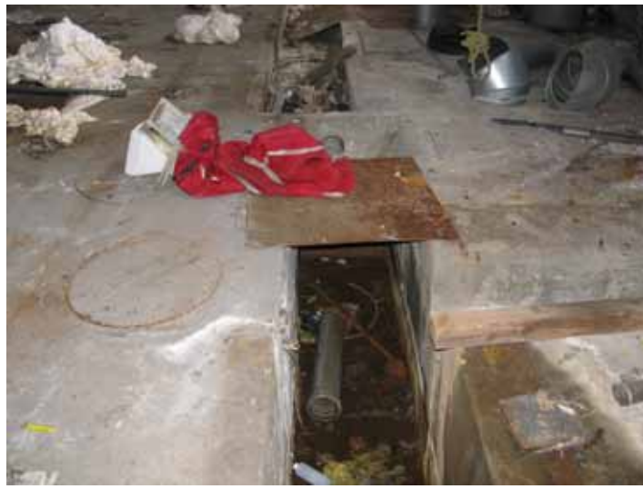
Typical trenches with sumps, staining, and standing water throughout the facility.
