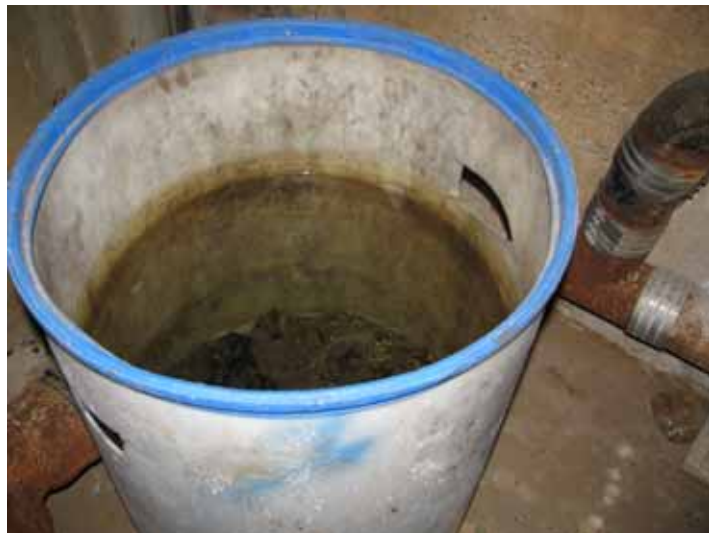
Open top drum with unknown contents in the southern basement.
