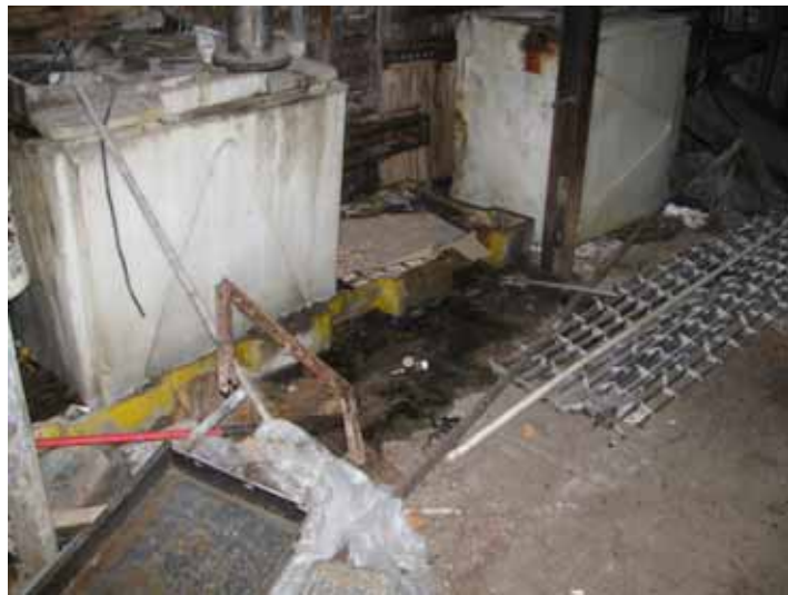
Overflowing chemical storage tanks on an overflowing spill containment pallet. Note the staining in front of the pallet.
