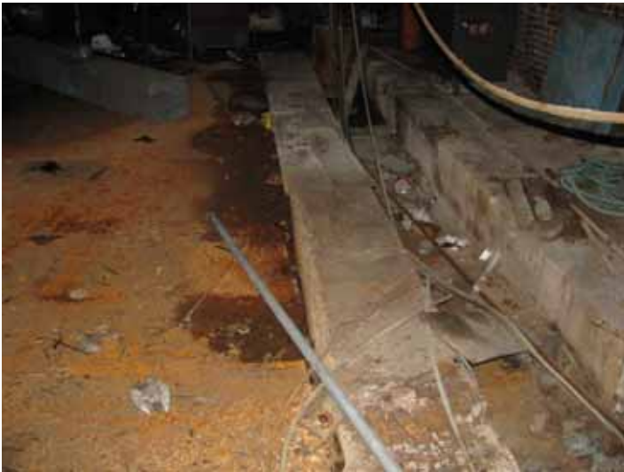
Stained trenches and road plates in the southern portion of the building.
