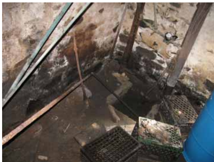
Alternate view of sump in central basement with drain pipes and a drum on the right side.
