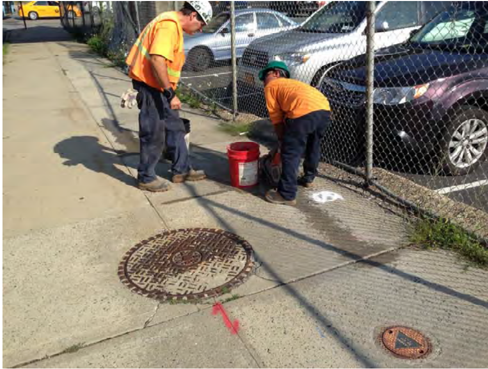
Photo 13: Saw cutting at soil boring SB-01, looking west. Existing well TRC-MW-4 is in foreground.
