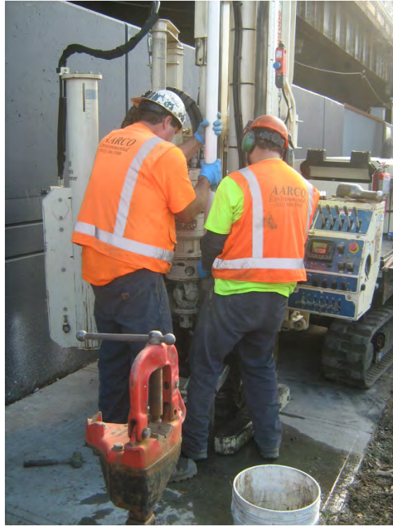
Photo 15: Installation of groundwater monitoring well DBMW-01 utilizing a hollow stem auger setup.
