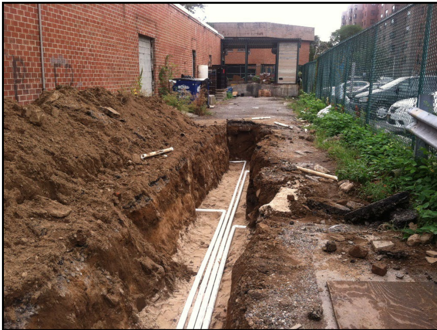
View of east end of the trench and piping and connections to wells AS-3 and AS-4 to the right, and wells SVE-6 and SVE-7 to the left. The trench was underlain with four inches of clean sand prior to installing the pipes.
