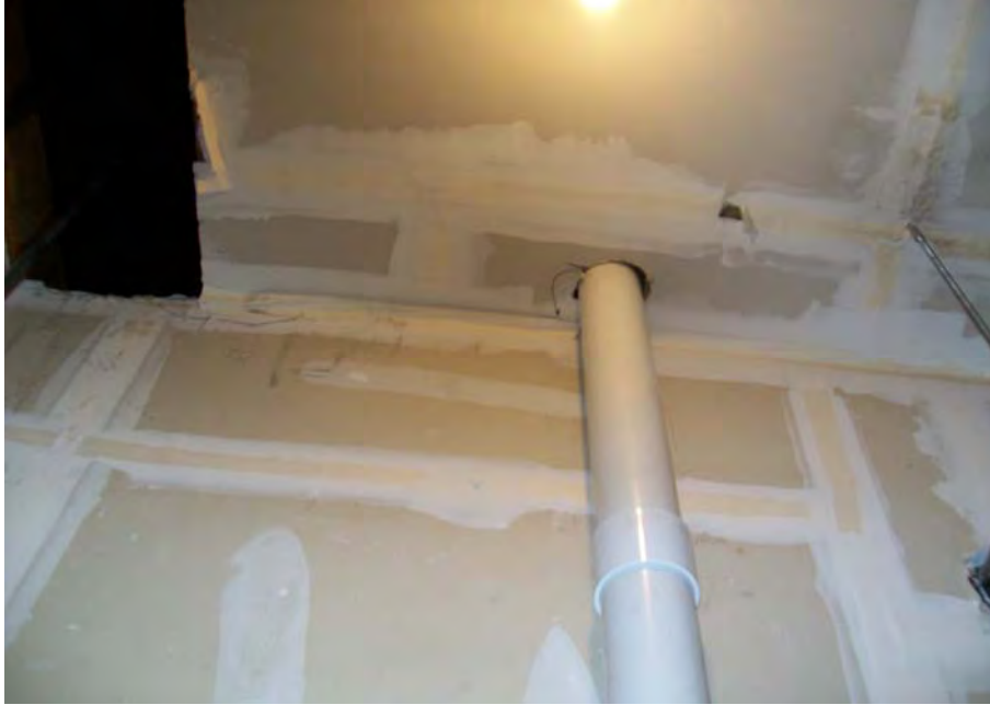
11. Suction piping continuing vertically to rooftop fan and system discharge point above first-floor utility closet and crawlspace entrance
