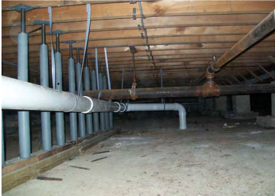
1. Suction point SP-1, looking north from MP-4
