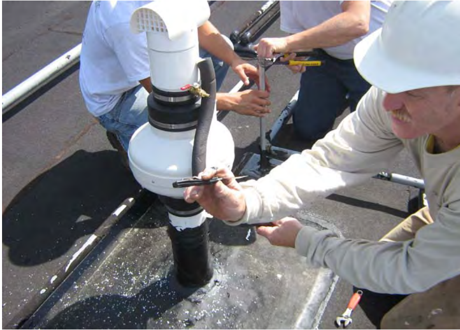
13. System fan with view of sample port and drain line
