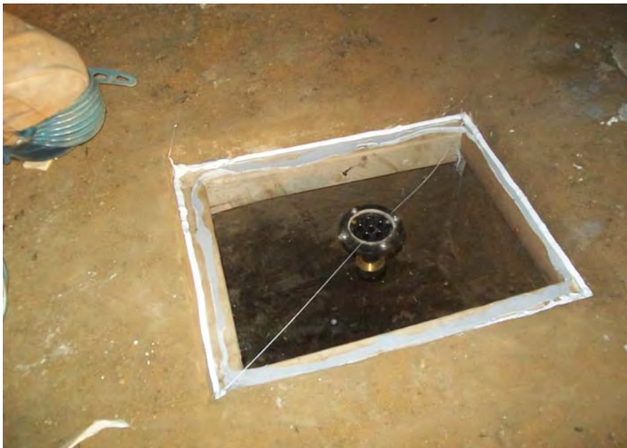
14. Sealed sump cover (recessed) with on-way Dranjer valve
