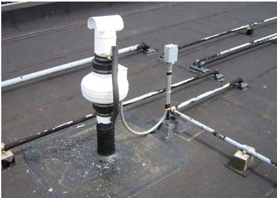
12. Exterior system features on south-central portion of building rooftop, immediately above the first-floor utility closet and crawlspace entrance
