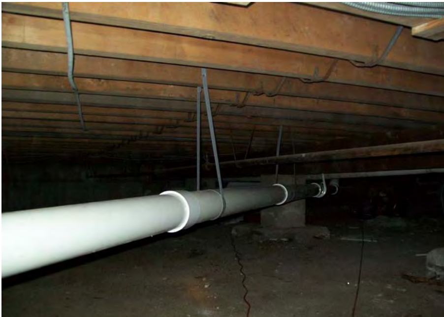
6. suction piping, looking southwest from drywall partition toward crawlspace entrance
