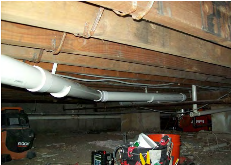
8. Suction piping, looking southwest toward crawlspace entrance from just northeast of entrance
