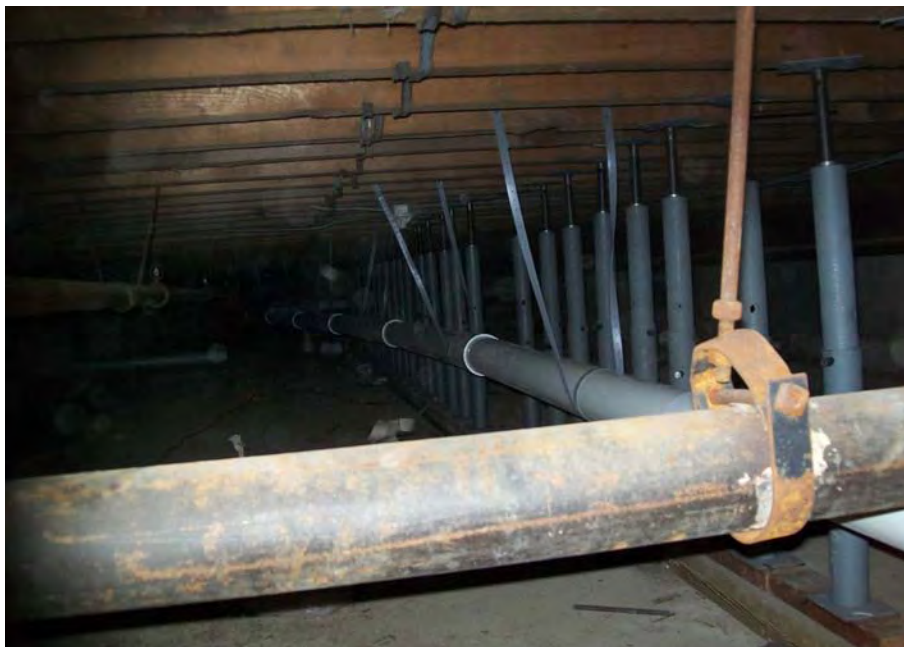
2. Suction piping, looking south from SP-1 toward SP-2
