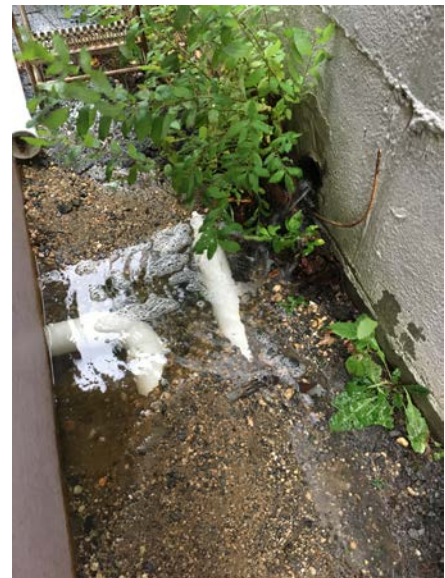
Water from roof drain ponding over horizontal well manifold
