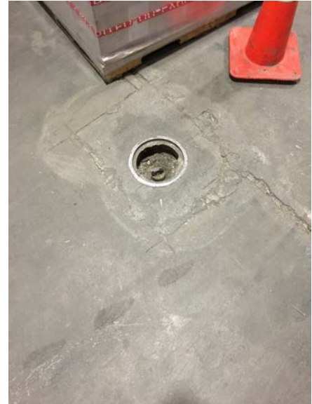
Missing well cap inside 1 Adams Blvd.
