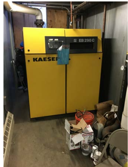
Blower in System #2 with faulty pressure gauge.
