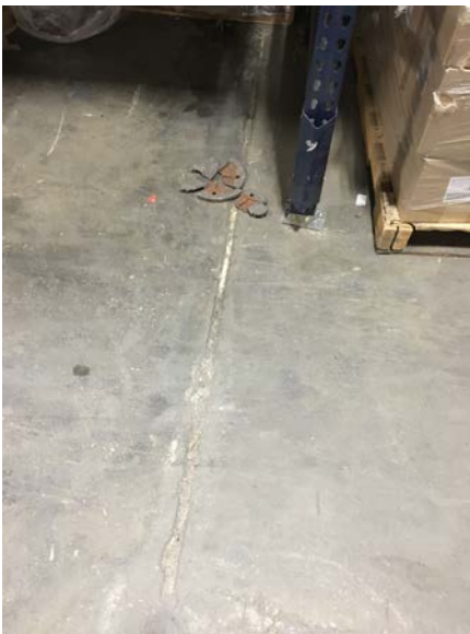
Well cap for MW-G
