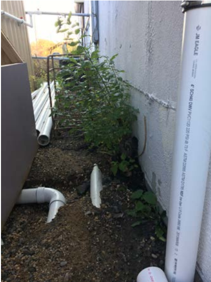
Erosion near SVE manifold
