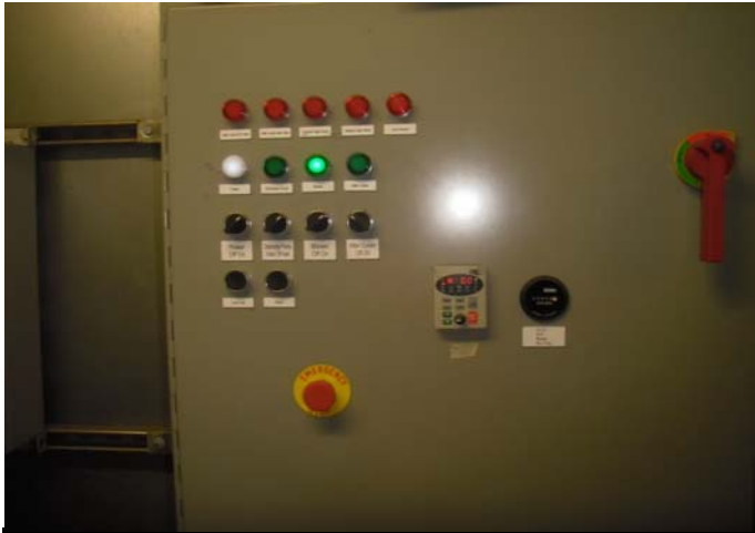
Picture 0026 - Both systems were running upon arrival with no alarms triggered.
