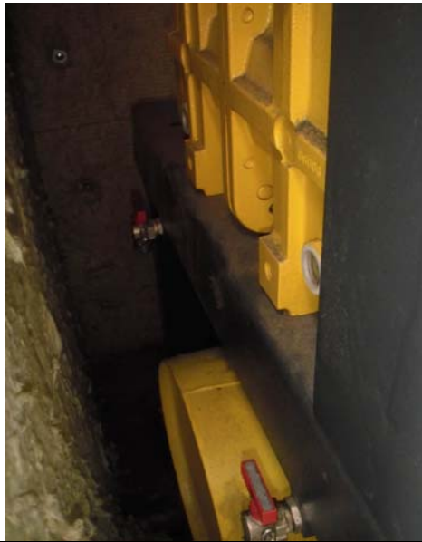
Picture 0031 - Oil levels were sufficient in each blower associated with System #1 and System #2.
