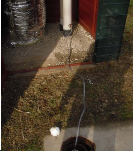
Picture 329- DDC-5 & DDC-6 condensate drainage valves were drained for 15 minutes.
