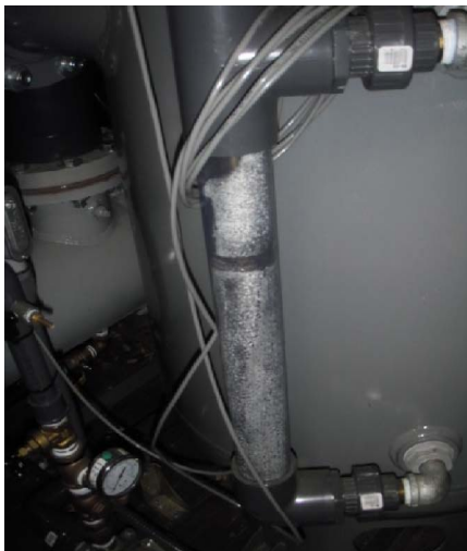
Picture 327- Condensation on the blower B-501 moisture separator was noted on the site glass.
