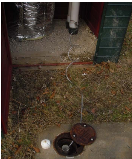
Picture 332- A condensation drainage valve was installed on the 4-inch injection line to DDC-6, with discharge hose to piezometer DDC-6-PD.
