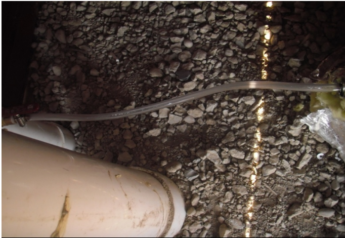
Picture 327- View of water discharging from the four (4)-inch injection line to the DDC-5-PS well.
