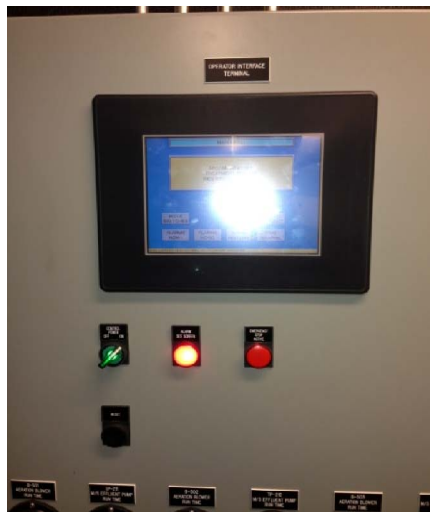
Picture 313- System was "Up" upon arrival with four (4) alarms triggered.
