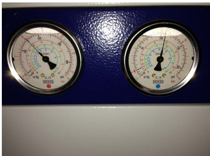
Picture 316- View of the Freon High Pressure and Freon Low Pressure gauges.
