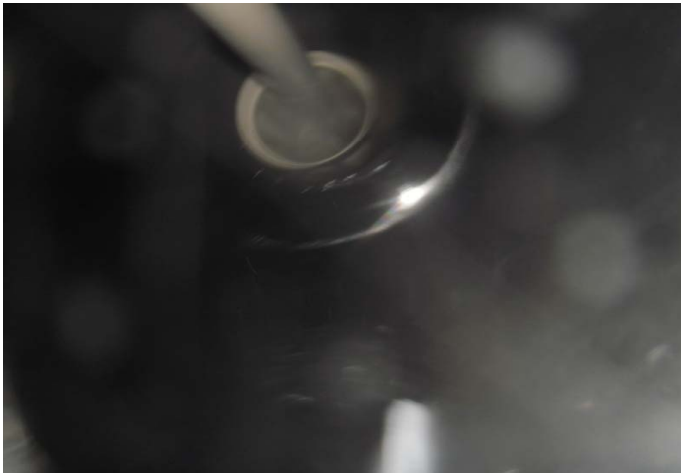
Picture 309- Bubbling was noted beneath the eductor head for DDC-5
