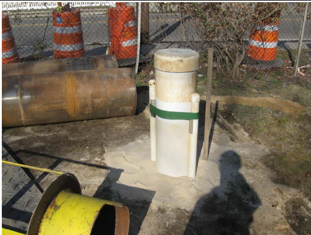
View of DDC-06 well and associated piezometers.
