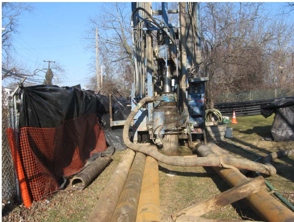
View of drill rig and drill rods at DDC-05. Note: poly along fence line.
