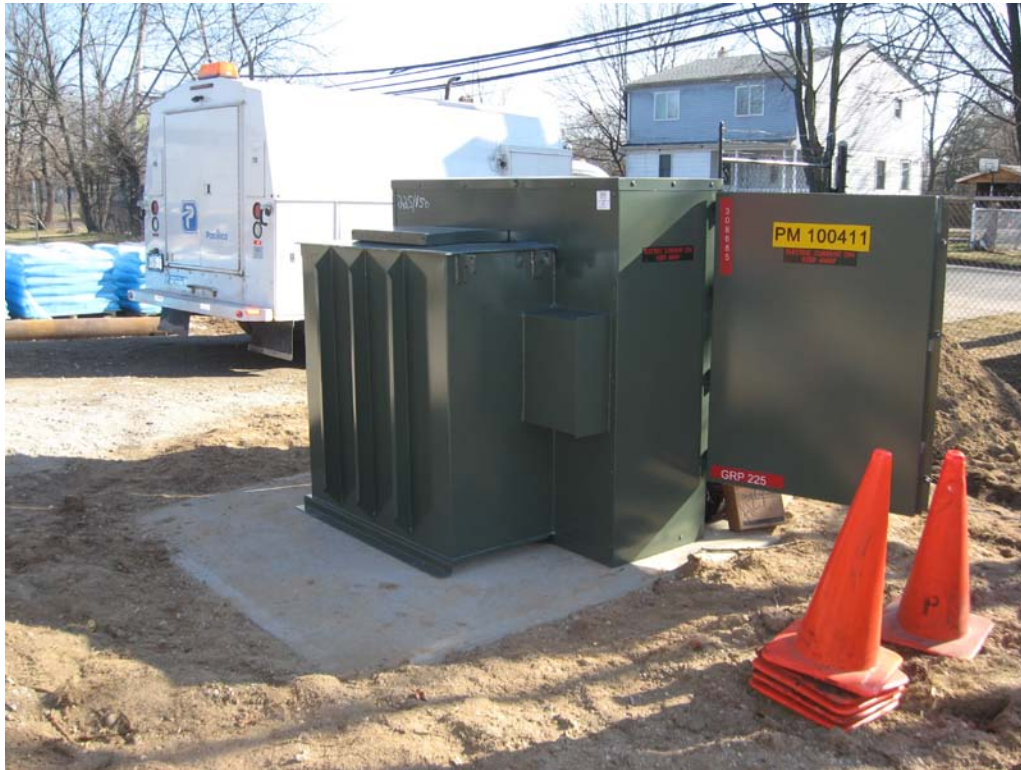
View of transformer on SCWA property.
