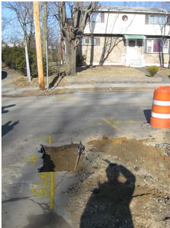
View of test hole and 4 Benjoe Dr. Note: Yellow paint on asphalt marks location of gas line.
