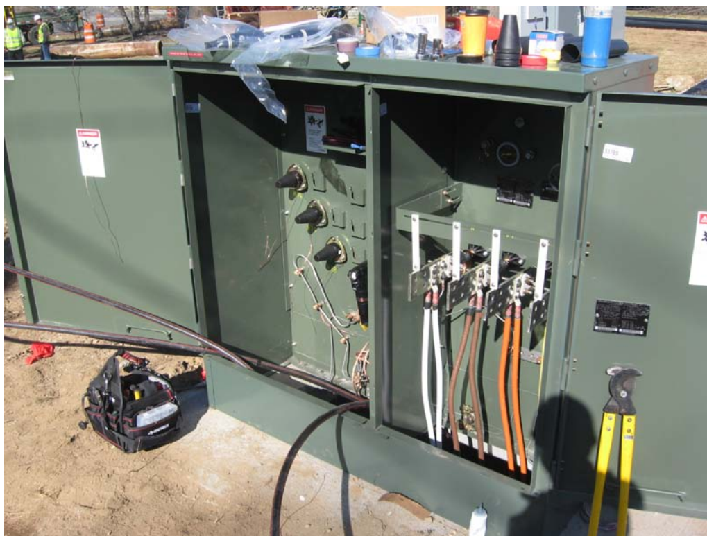
View of transformer interior and connections.
