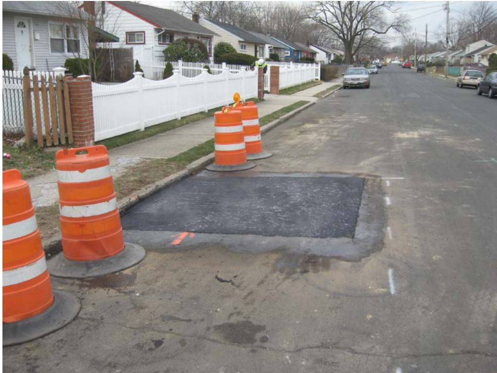
Temporary asphalt patch at DDC-10.
