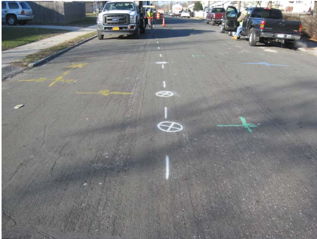
Test hole markouts (white circles) and 6-in. supply/return line markouts (white dash).
