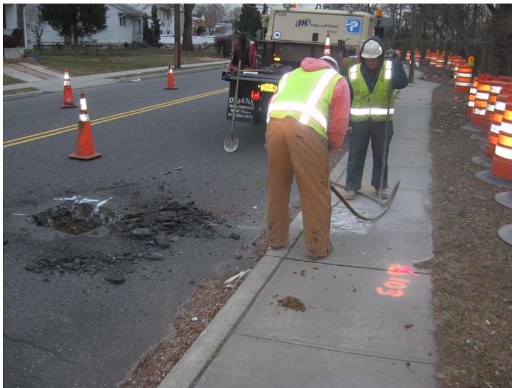
Posillico jack hammering concrete sidewalk for utility test hole along Albany Ave, looking north.
