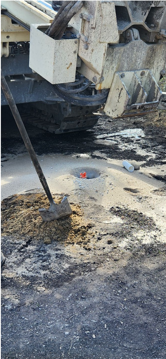
At left: MW-3A installed, prior to removal of excess cuttings and placement of protective manhole.
