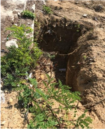
Hole next to slab
