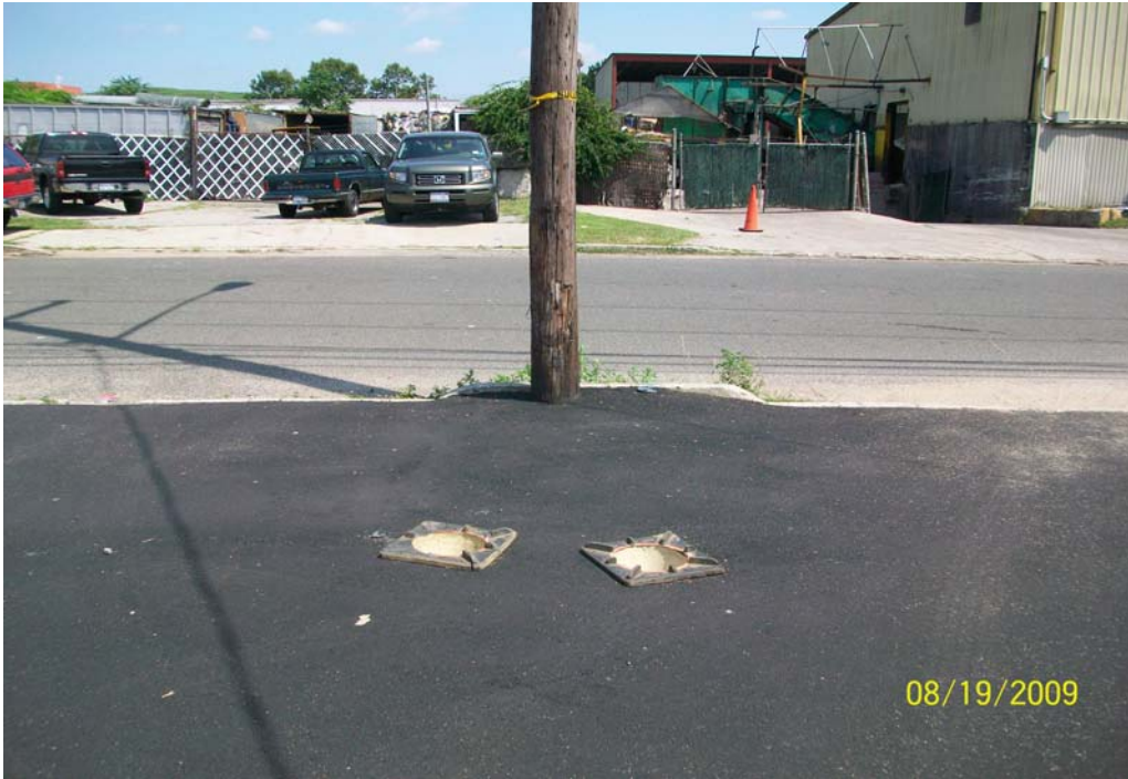
100_1192.jpg - Missing water meter covers in front of 50/60 Dale St.
