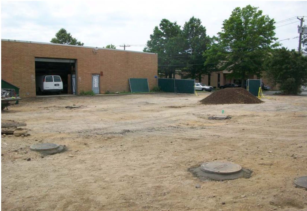
100_0927.jpg - Raised manhole covers at 51 and 61 Cabot St.
