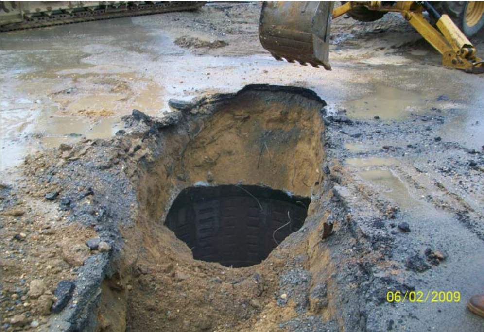
004.jpg - DS-6 partially abandoned, 61 Cabot St.
