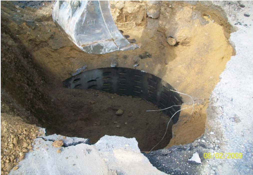
001.jpg - DS-3 partially abandoned, 51 Cabot St.
