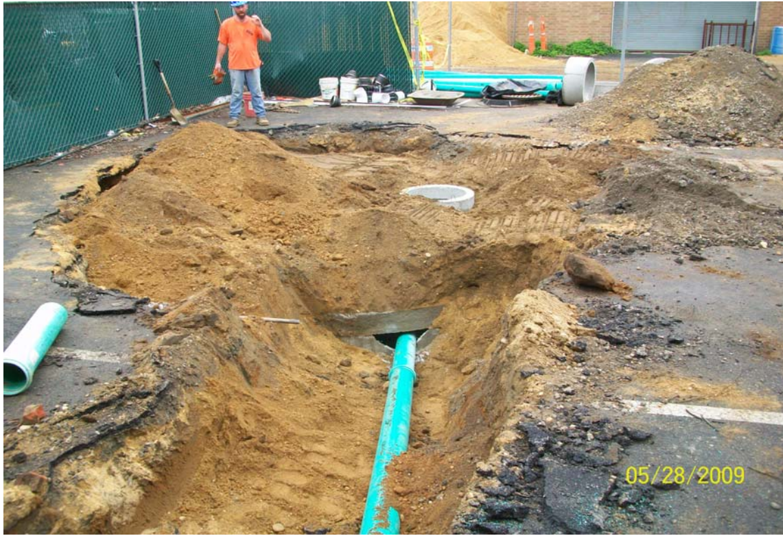
100_0723.jpg - Eastern most roof drain, 61 Cabot St., redirected from DS-4 to PDS-3
