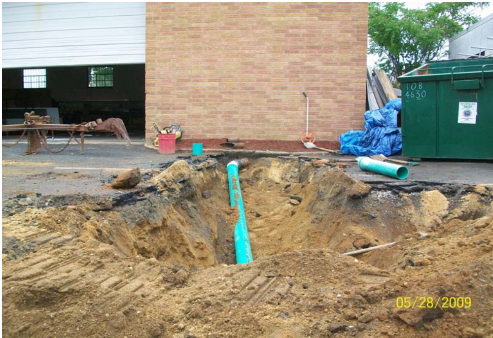
100_0722.jpg - Eastern most roof drain, 61 Cabot St., redirected from DS-4 to PDS-3
