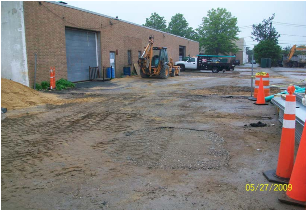
100_0699.jpg - CP-7 completely abandoned, 51 Dale St.
