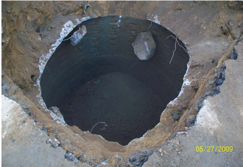
100_0696.jpg - Dome of CP-7 broken into structure, 51 Dale St.
