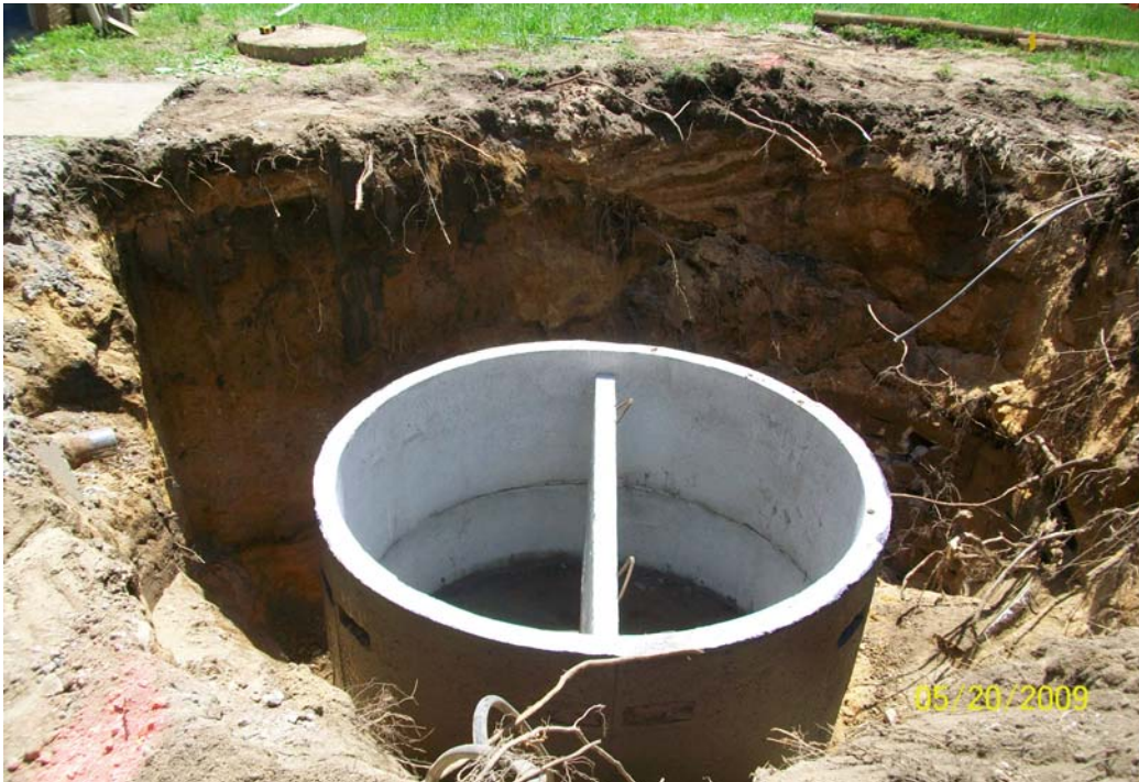
100_00645.jpg - PST-4 installed with baffle wall
