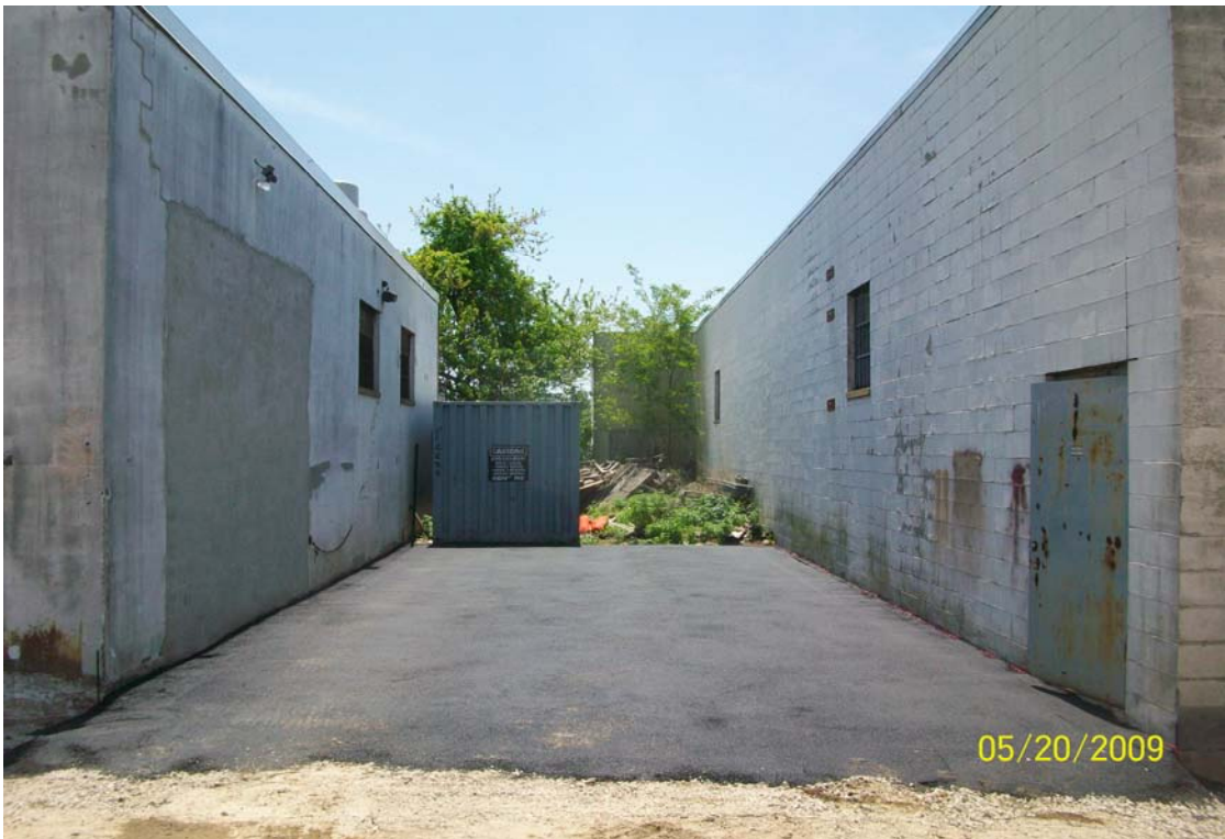
100_00644.jpg - South alleyway completely paved with a 3" binder course and a 2" wear course
