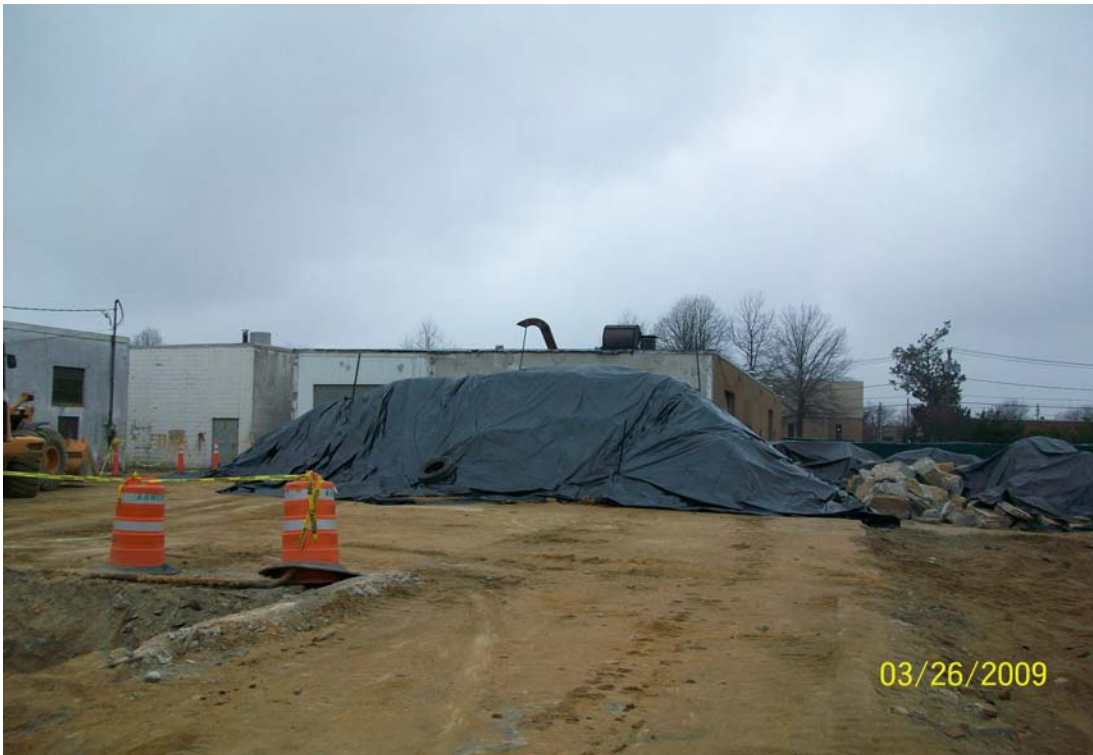
100_00226.jpg - Mt. Spectrum, hazardous waste soil stockpile
