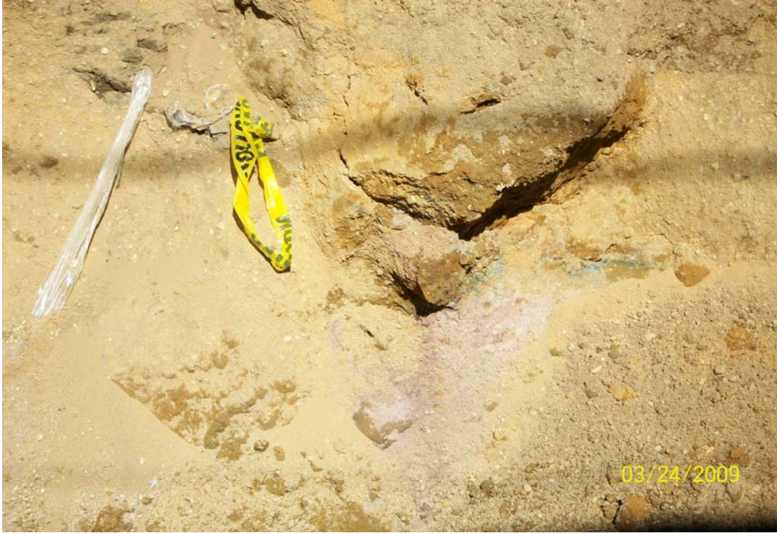
100_00179.jpg - Red and green soil staining on face of excavation.
