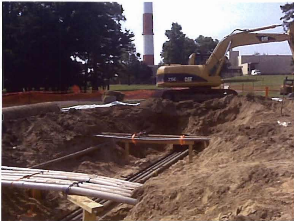
Photograph 3 – Exposed Waste Transfer Lines beneath braced active underground utilities
