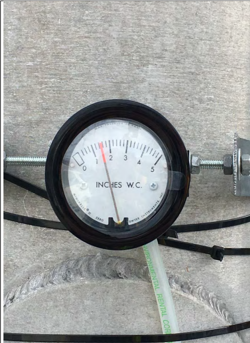
Photograph: 13 Installed Vacuum Gauge (Minihelic)
