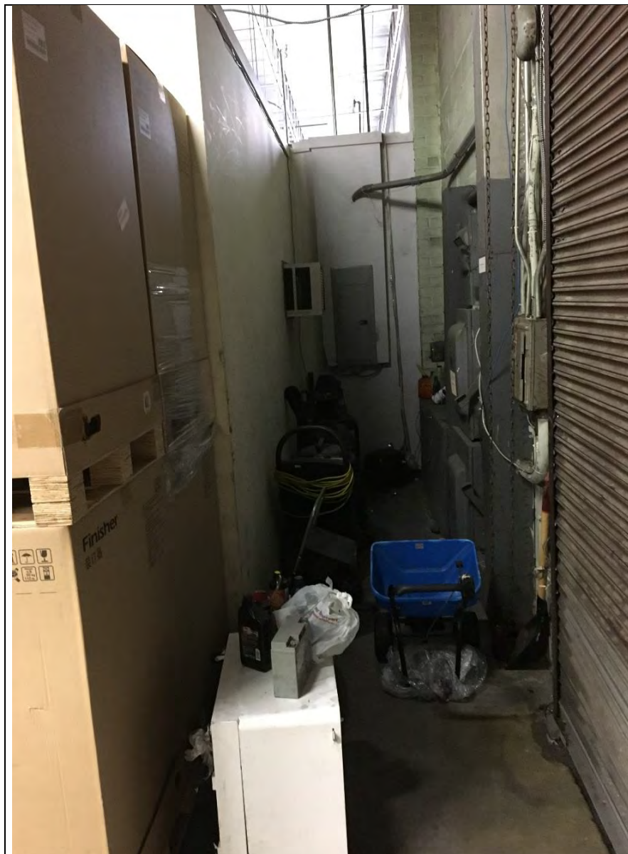
Photograph: 16 Electrical Panel Supplying Power To Fan
