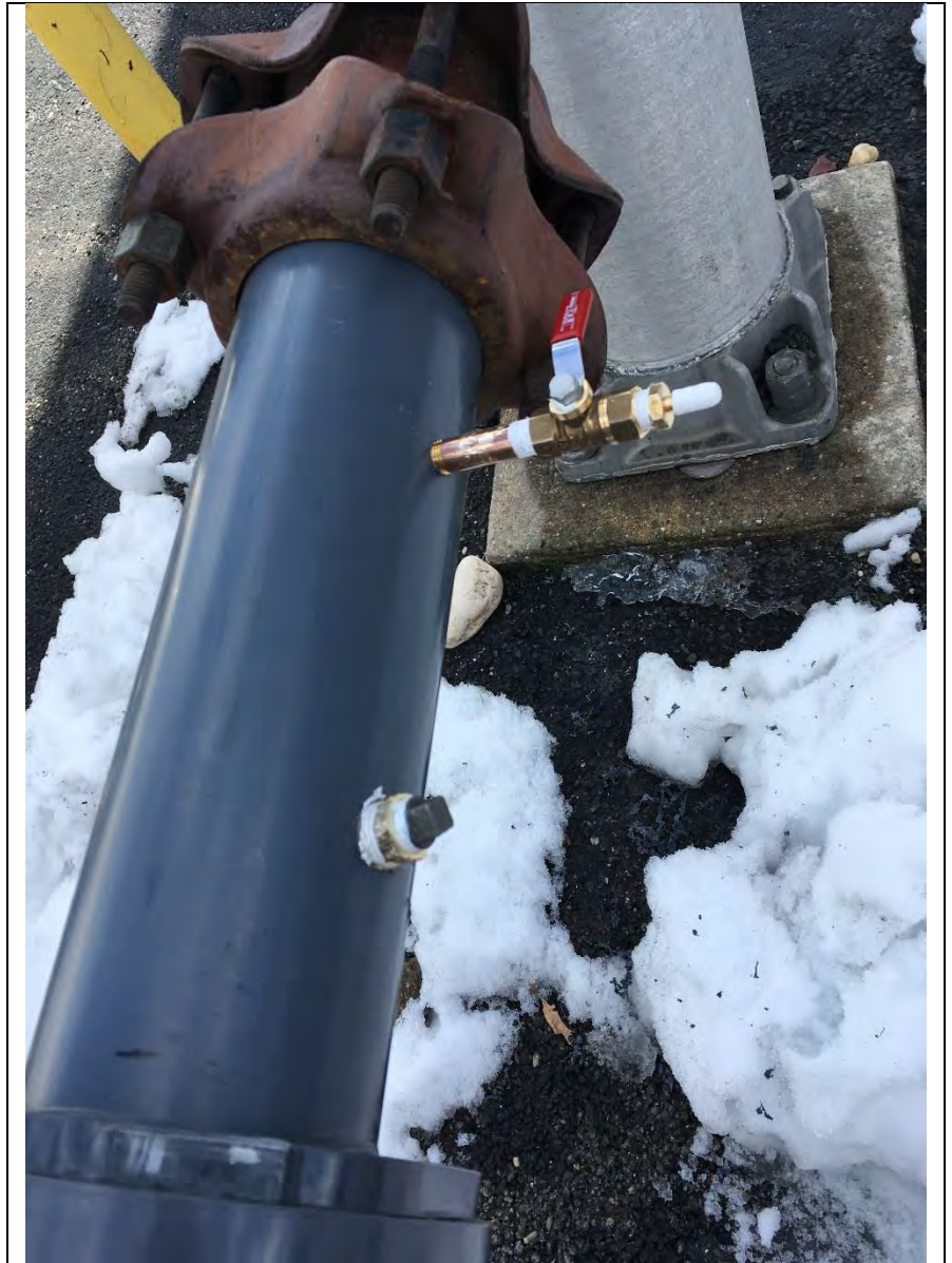
Photograph: 12 Installed Sample Port and Flow Measurement Port
