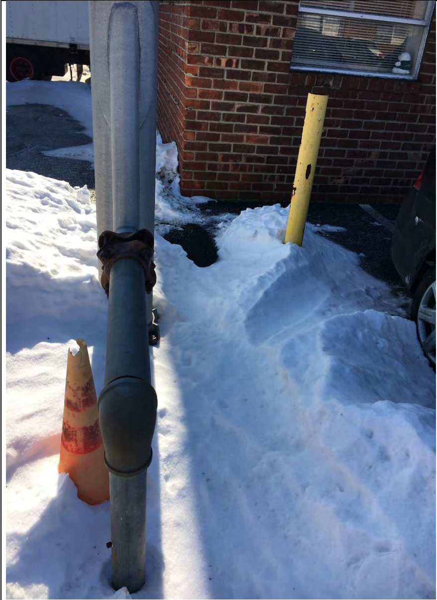
Photograph: 1 Sub Slab Venting System Stack Piping To Be Modified
