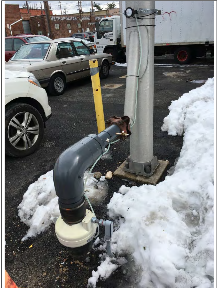
Photograph: 14 Installed Sample Port, Flow Measurement Port and Vacuum Gauge
