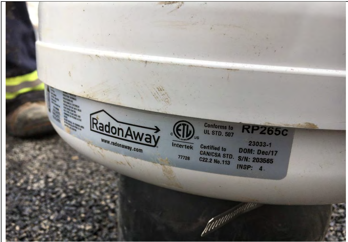
Photograph: 7 | Installed Fan Brand/Model/Serial Sticker
