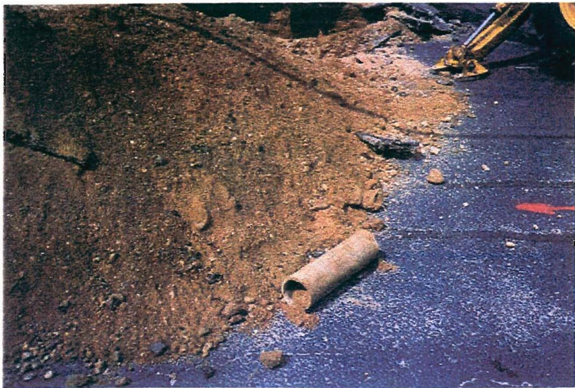
Piece Of The 5" Drain Pipe That Was Connected To Dry Well
