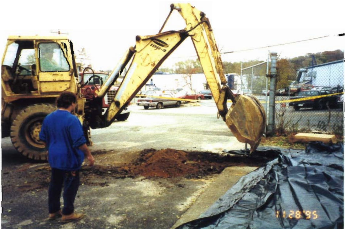
PHOTOGRAPH # 2 : Excavation Activities Begin, Note Well in Center of Excavation. Looking East.
