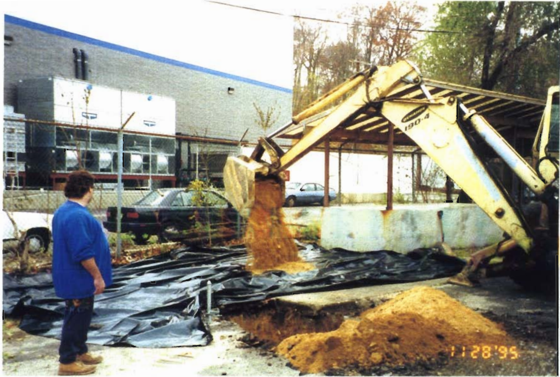
PHOTOGRAPH # 3 : Placement of Soil on Liner. Photocircuit Building in Background. Looking South.
