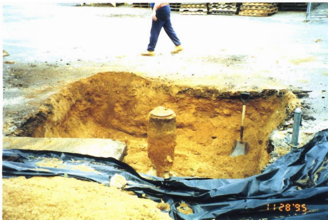
PHOTOGRAPH # 6 Three Foot Deep by Ten Foot Square Excavation Completed. Looking North.
