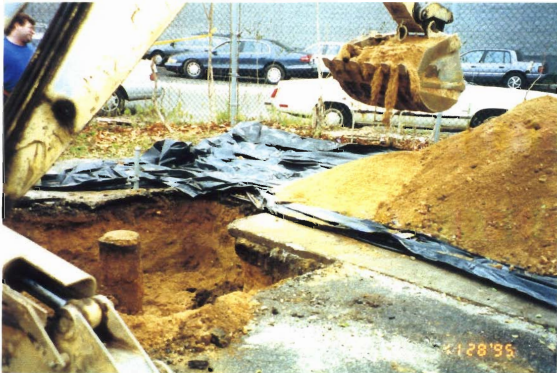
PHOTOGRAPH # 4 : Excavation Nearing Completion. Looking East. Note Monitoring Well in Center of Excavation.
