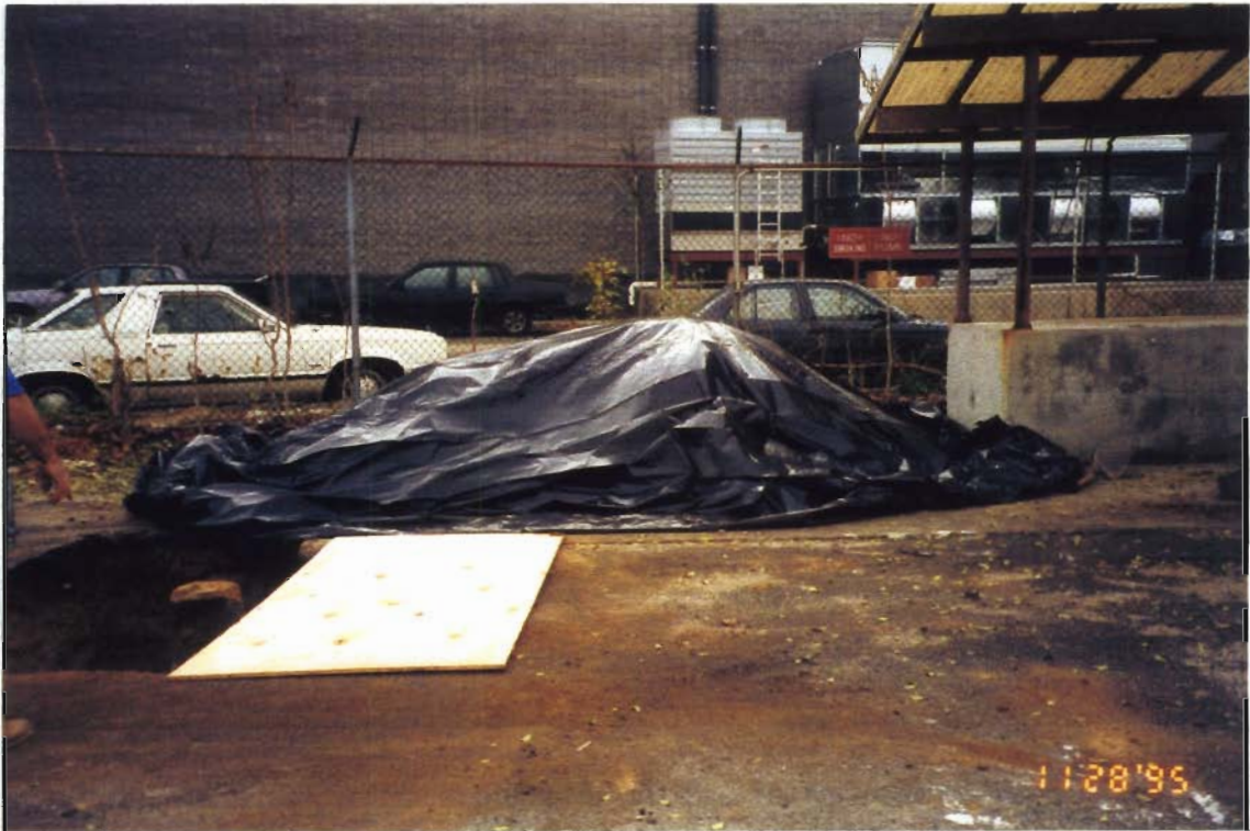
PHOTOGRAPH # 11: Waste Pile Covered with Sheeting. Large Rocks Used to Secure Top.
