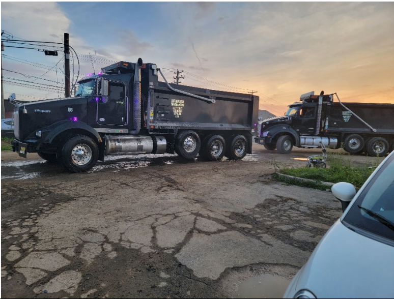
Photo 3: Looking northeast, Pratt cleans truck wheels exiting the site prior to tracking pads for dust mitigation and sediment track out control.
