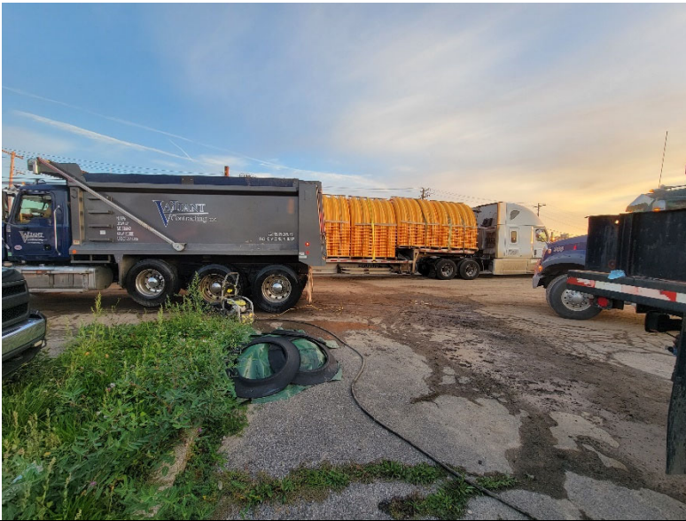
Photo 3: Looking northwest, Pratt cleans truck wheels exiting the site prior to tracking pads for dust mitigation and sediment track out control. Pratt receives delivery for drainage basin structures.
