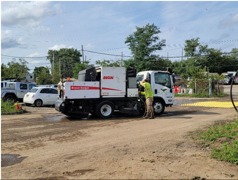
Photo 1: Looking southwest, Pratt uses broom badger to sweep along Commerce Place and New South Road, as well as the stabilized construction entrance and onsite asphalt parking area. Pratt cleans tracking pads using power washer.
