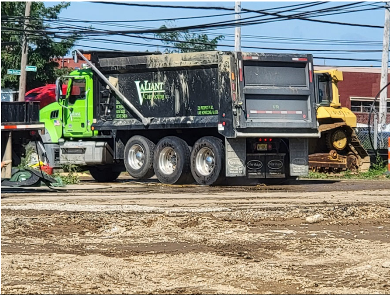
Photo 3: Looking northwest, Pratt cleans truck wheels exiting the site prior to tracking pads for dust mitigation and sediment track out control.
