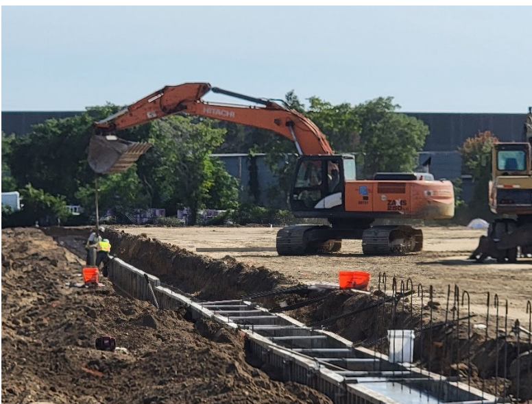
Photo 4: Looking south Ruttura and Pratt continue excavation and foundation formwork along the eastern and southern side of the building footprint.
