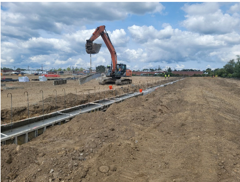
Photo 4: Looking north, Ruttura and Pratt continue excavation and foundation formwork along the eastern and southern side of the building footprint.
