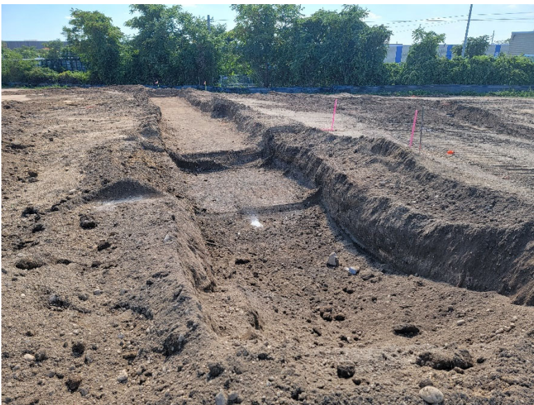
Photo 4: Looking west Ruttura & Pratt continue excavation for foundation formwork along the southern side of the building footprint.
