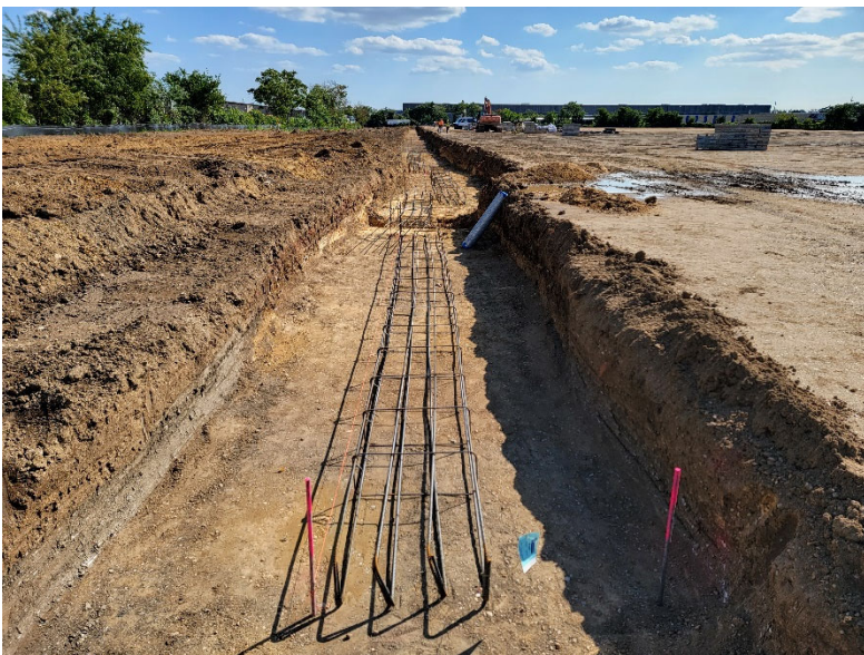
Photo 4: Ruttura & Pratt begin excavation for foundation formwork along the eastern side of the building footprint.
