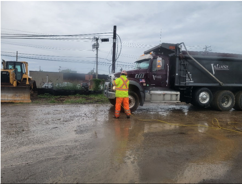
Photo 3: Looking north, Pratt cleans truck wheels exiting the site prior to tracking pads for dust mitigation and sediment track out control.
