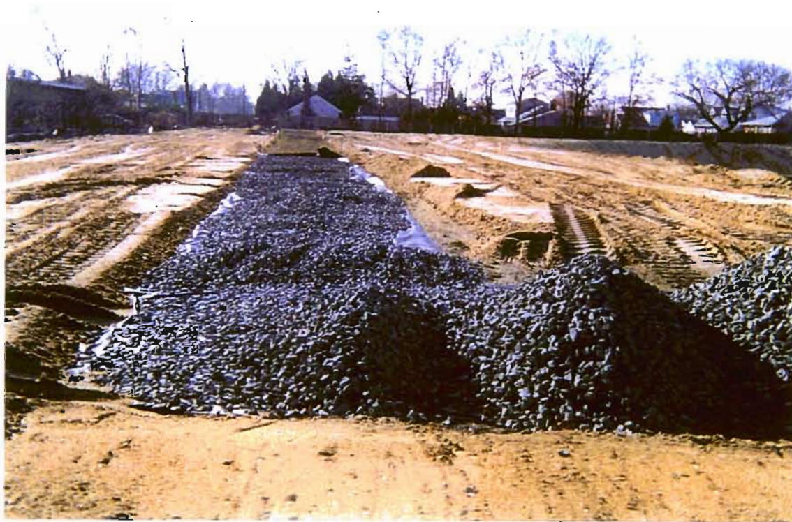
EASTERN ACCESS ROAD CONSTRUCTION, LOOKING SOUTH. SOIL COVER MOSTLY COMPLETE ON SIDES
