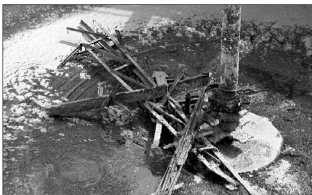
Lack of preventive maintenance may cause violations.
