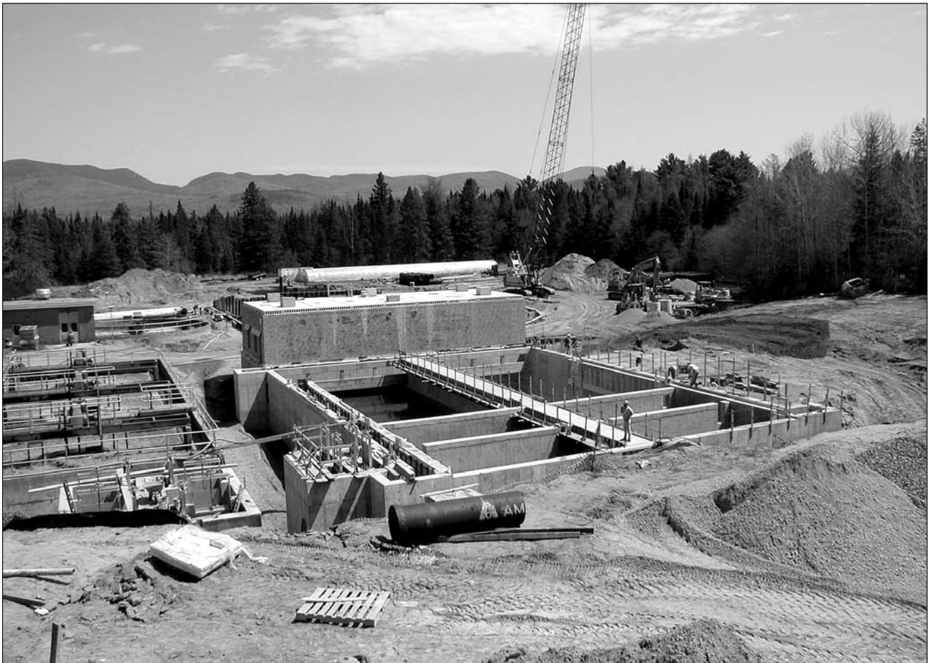
Sometimes a plant upgrade is needed to maintain SPDES compliance. (Lake Placid)
