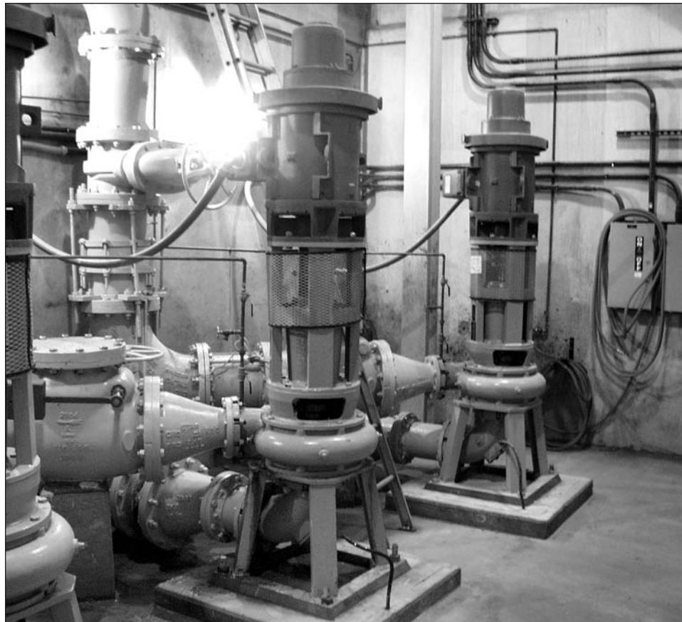
New and more efficient pumping (Herkimer County Sewer District)
