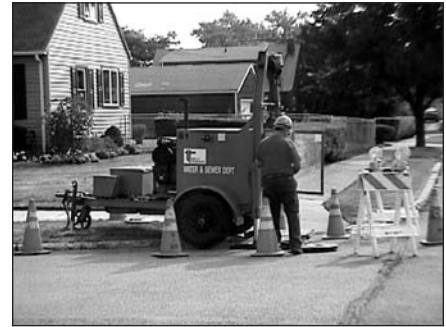
Proper maintenance of the collection system is critical for optimum system performance. (Town of Tonawanda)
