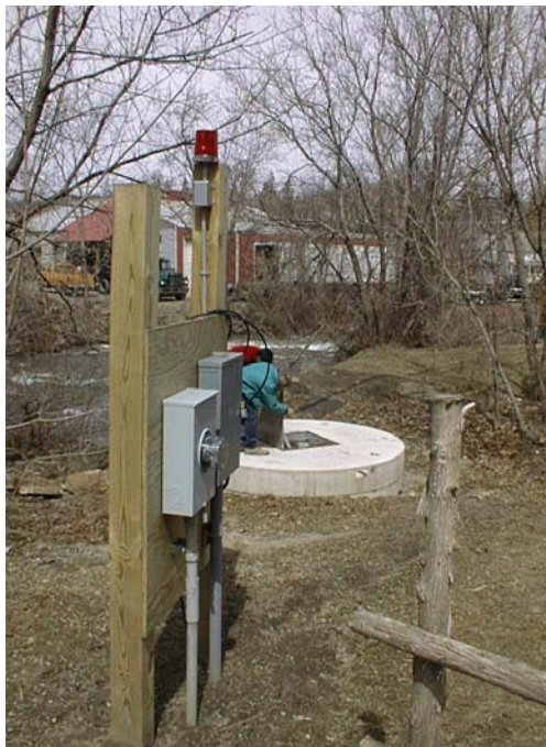
Collection system CSO (outfall 003) Alarm light and power source for sampler
