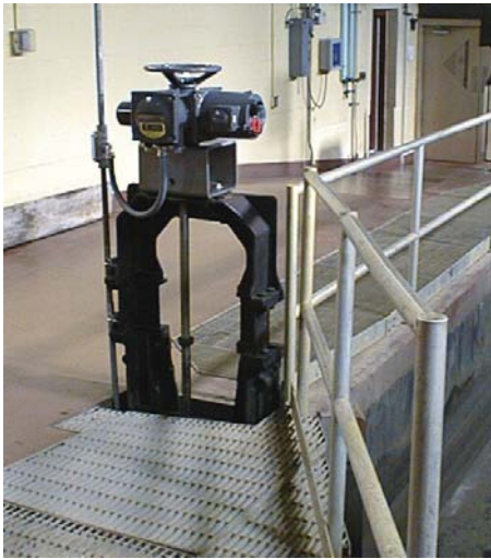
Programable flow diversion gate for stormwater storage.
