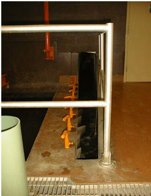
Adjustable vanes for grit chamber help direct flow evenly across the tank. Vanes are throttled closed as flow increases.
