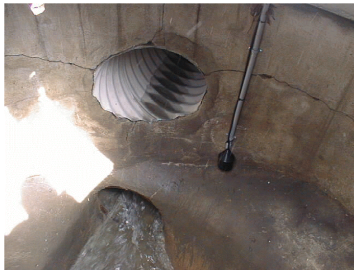
Alarm switch inside manhole of collection system CSO.
