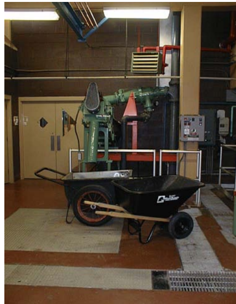
Cyclone degritter and grit buggies. Cyclone pressure must be kept at a minimum 7-8 psi.
