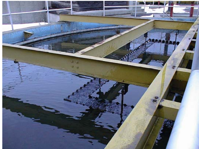
Secondary clarifier during simulated wet weather event.
