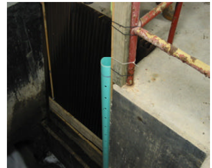
Influent channel after plant staff added an additional 16 inches of storage
